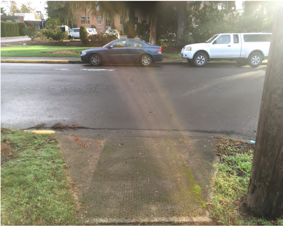
N Meridian Street/E Franklin Street looking east from the northwest quadrant; No curb ramp is provided on the east side & parking is not restricted
