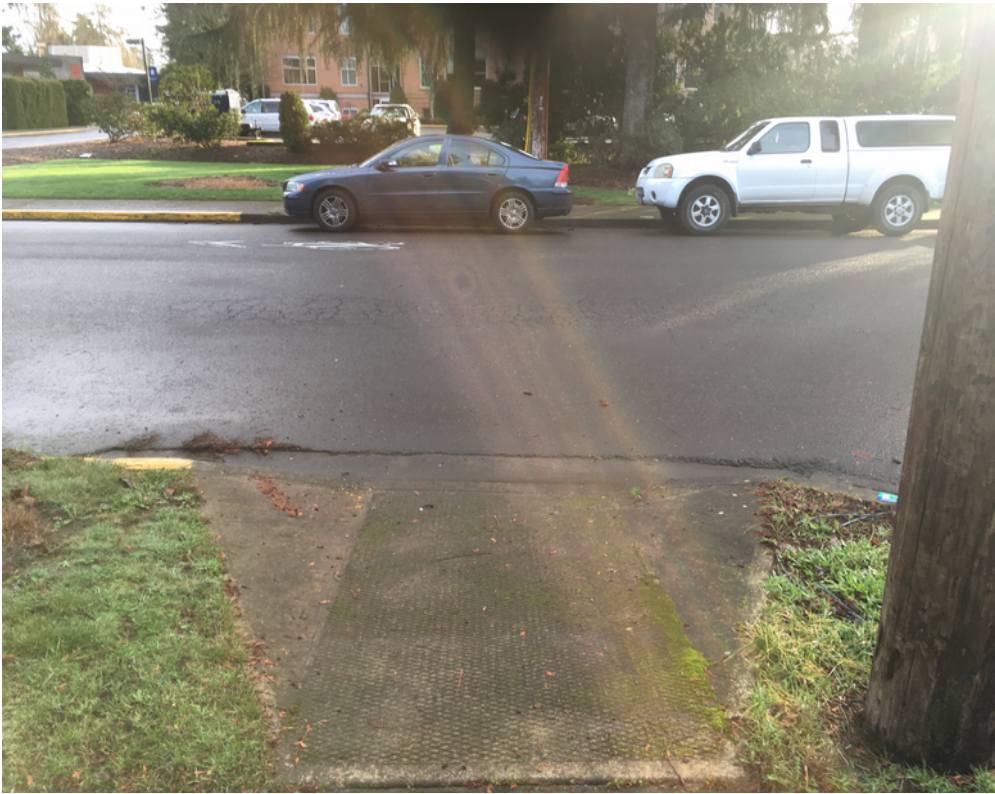
N Meridian Street/E Franklin Street looking east from the northwest quadrant; No curb ramp is provided on the east side & parking is not restricted
