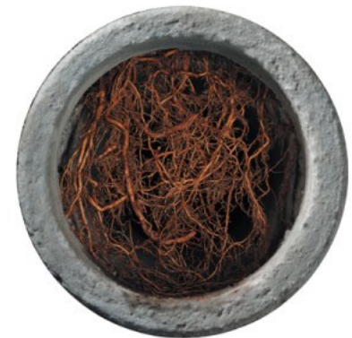
Root intrusion in service line
