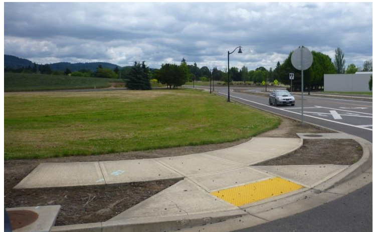
ADA Compliant Curb Ramp with No Connections
