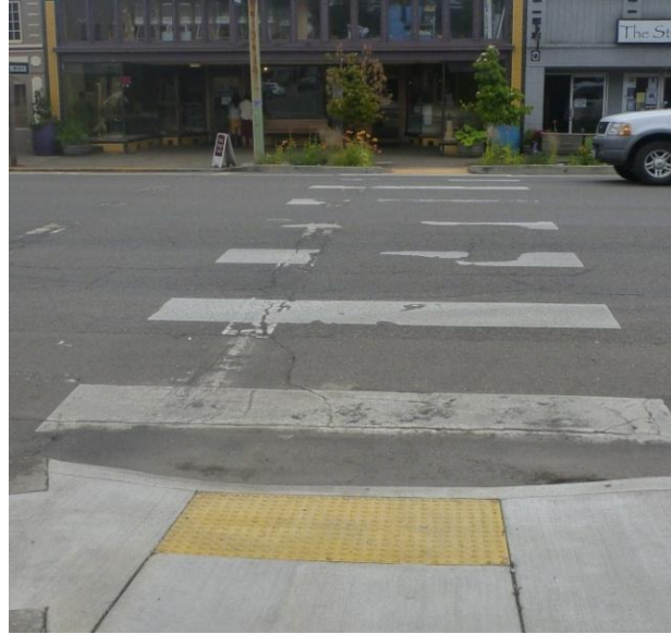
Faded Crosswalk in Downtown Newberg
