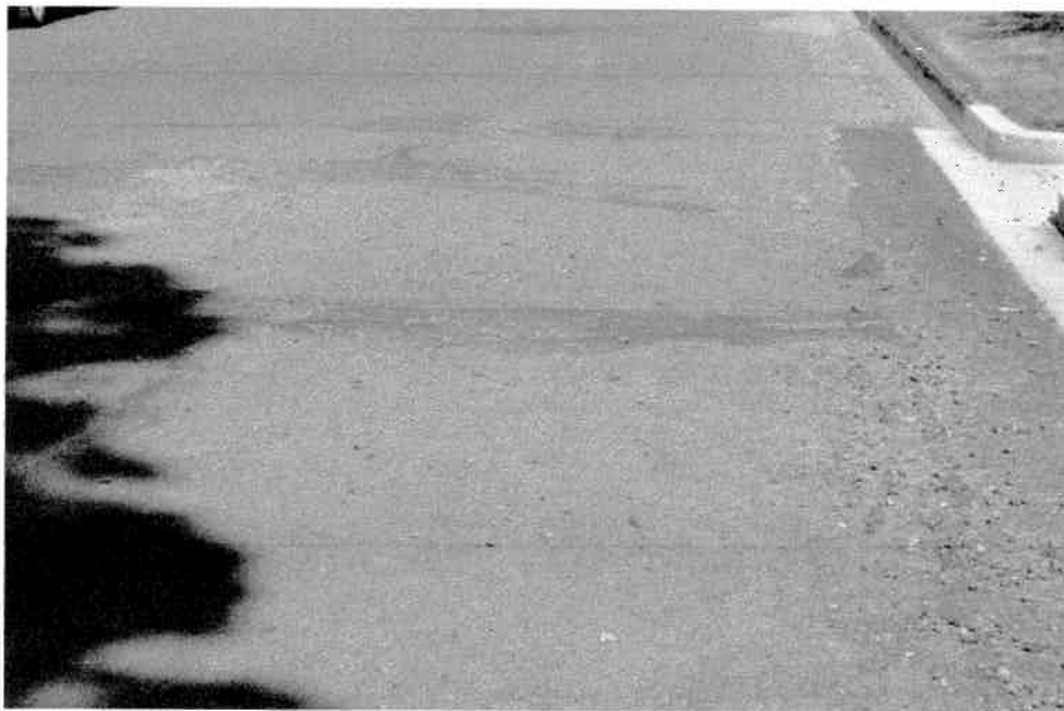
Picture #4: Potholes and road bed debris at N. Howard St. entrance to new parking lot.
