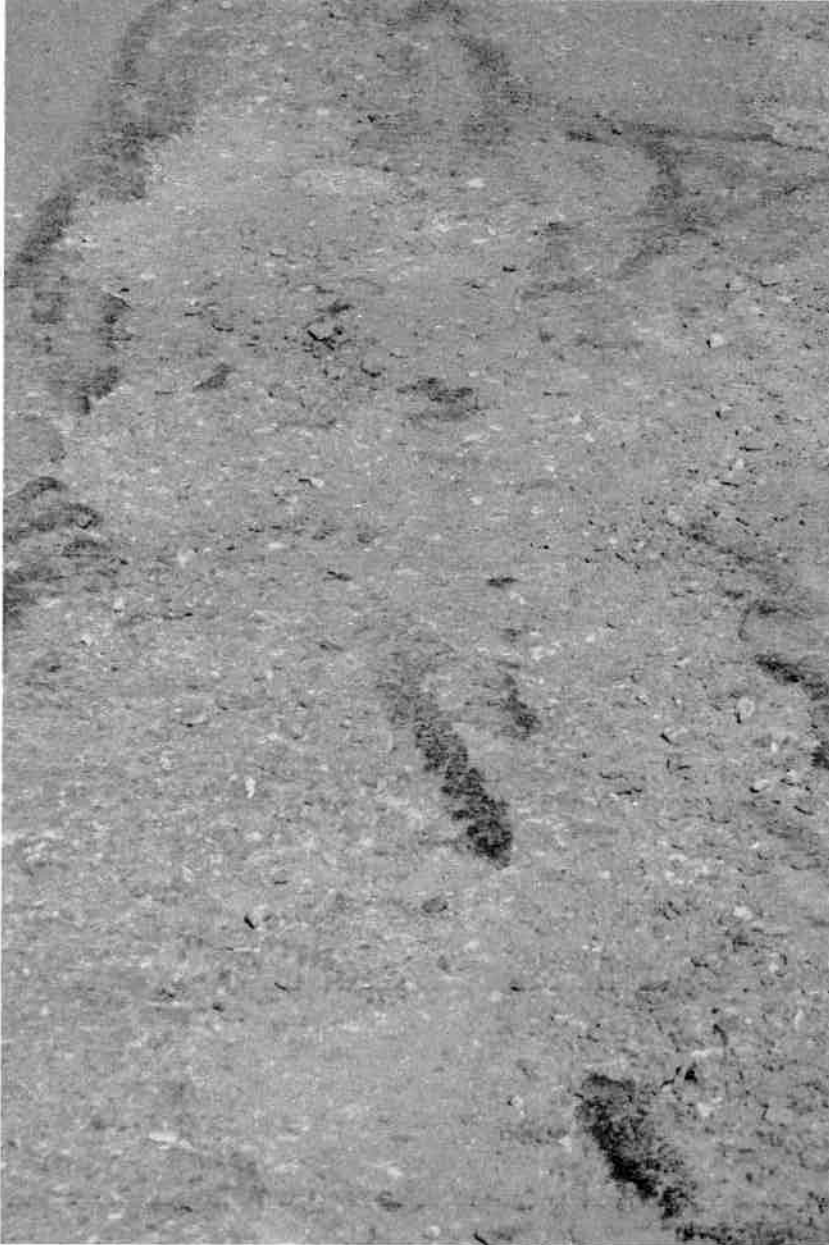
Picture #2: Close up of Picture #1 pothole. Note that the gravel roadbed is becoming exposed and gravel is working loose as obstructions on the street.
