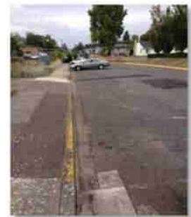
Newberg: Faded striping
