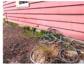
Faucet, West side, 808
