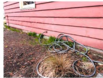
Faucet, West side, 808
