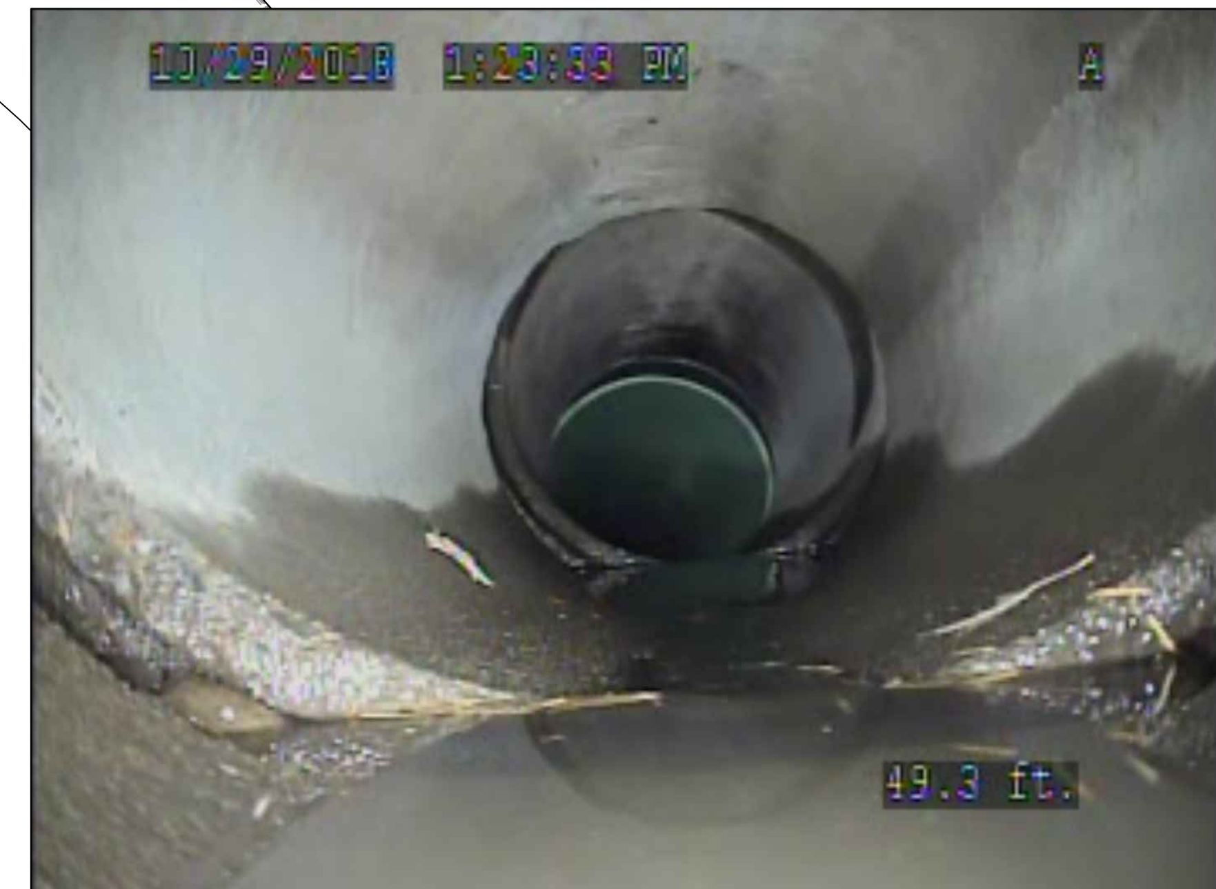
FIG. 1: SEPARATED JOINTS IN EX. STORM PIPE
