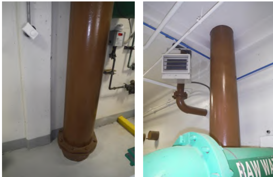
Figure 3.19 – Vertical Pipe without Lateral Restraint
