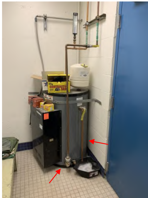
Figure 3.45 – Water Heater Tank not Adequately Restrained
