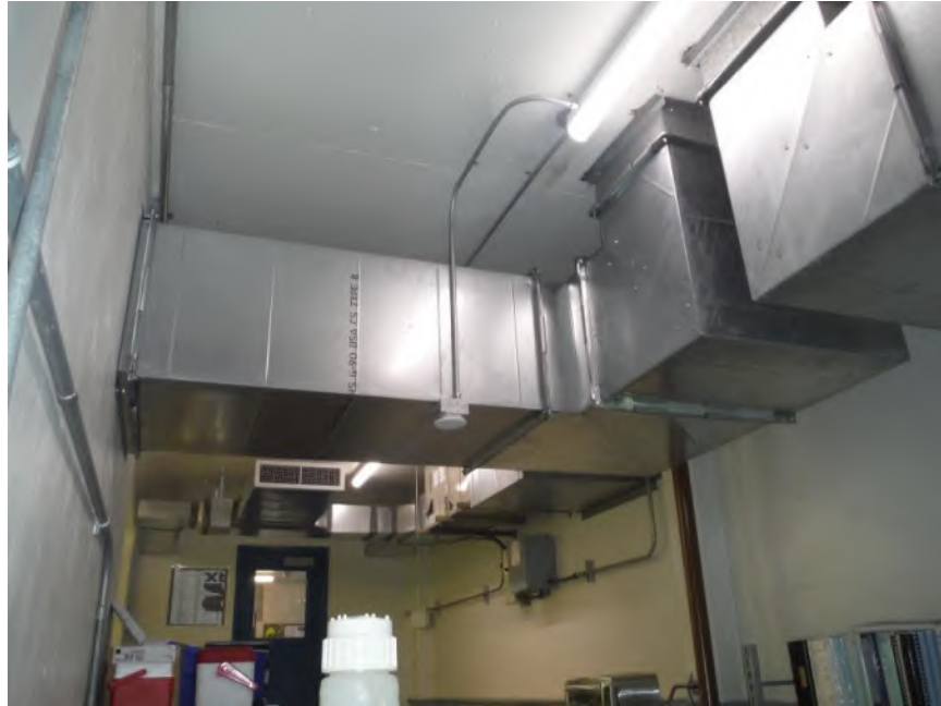
Figure 3.24– Mechanical Ducts not Braced to Structure
