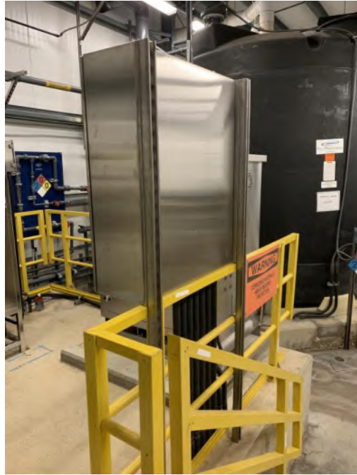
Figure 3.89 – Control Panel not Adequately Braced
