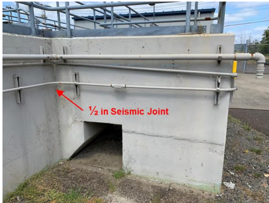
Figure 3.50 – Sedimentation Basins Effluent Structure (Outlet Basin Structure)
