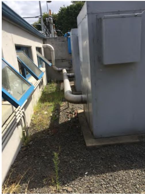
Figure 3.65 – Air Scour Piping from Blowers to Filter Gallery without Adequate Flexibility to Accommodate Differential Movement
