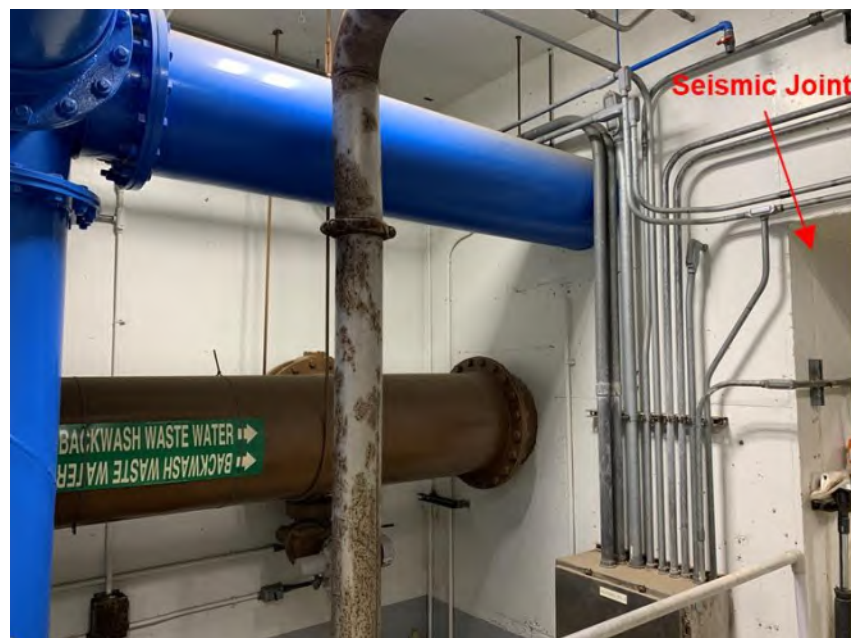
Figure 3.62 – Finished Water Sample Pipe and Filter Backwash Pipe Cross Seismic Joint without Adequate Flexibility
