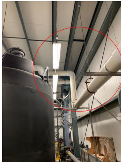
(b) Unbraced Piping Inside the Building
