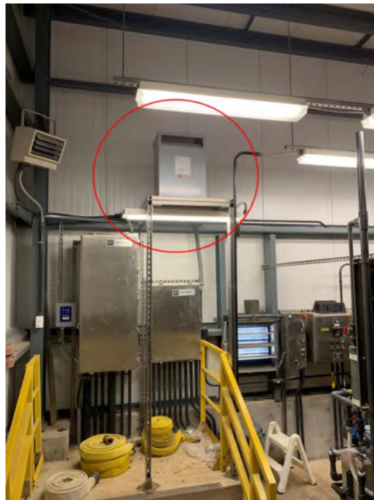
Figure 3.90 – Transformer not Adequately Braced
