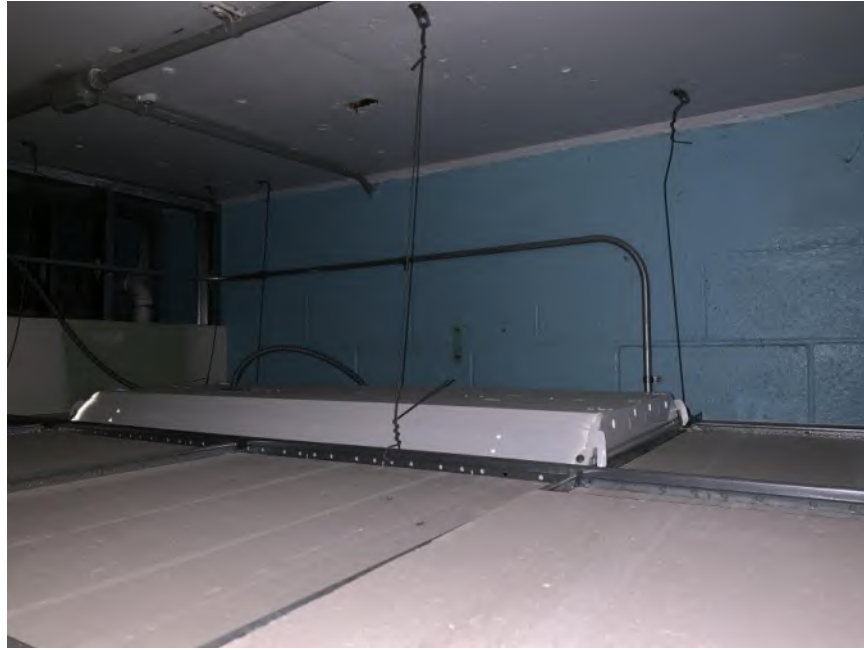
Figure 3.46 – Light Fixture Supported by Ceiling Grid
