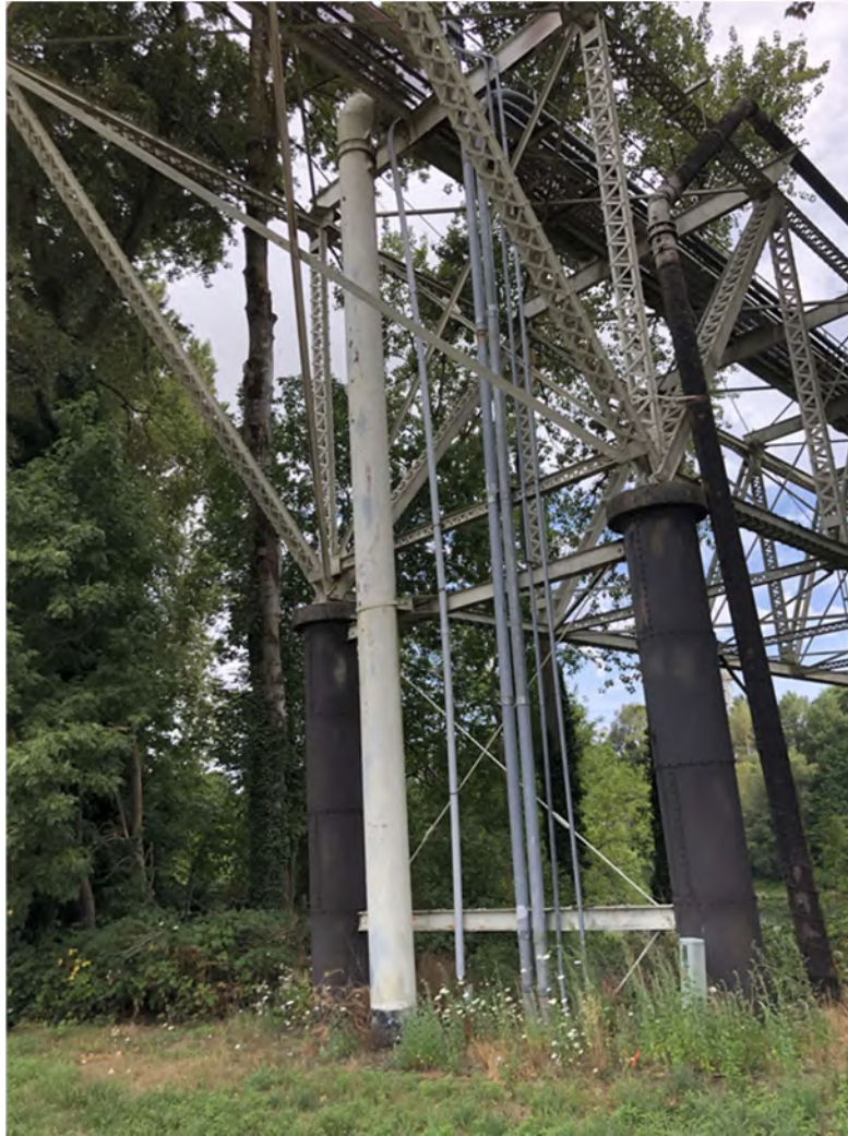
Figure 2. 24-inch Water Transmission Main
