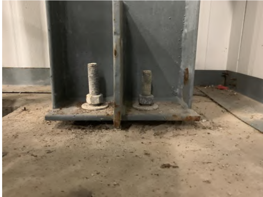
Figure 3.79 – UngROUTed Base Plate and Nuts on Anchor Rods not Tight
