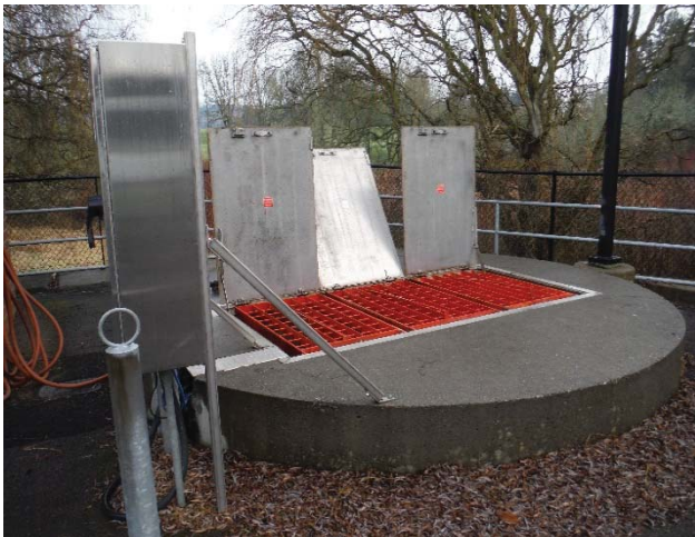
Fernwood Lift Station
