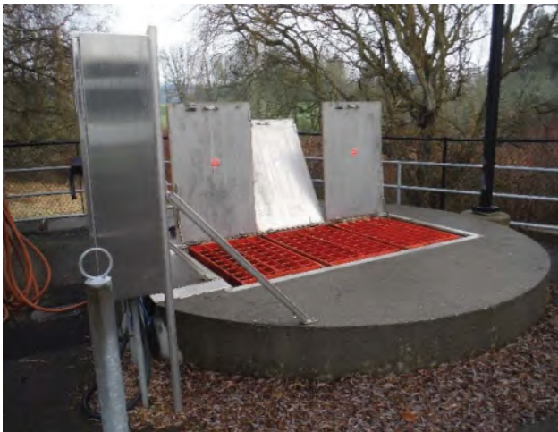
Fernwood Lift Station
