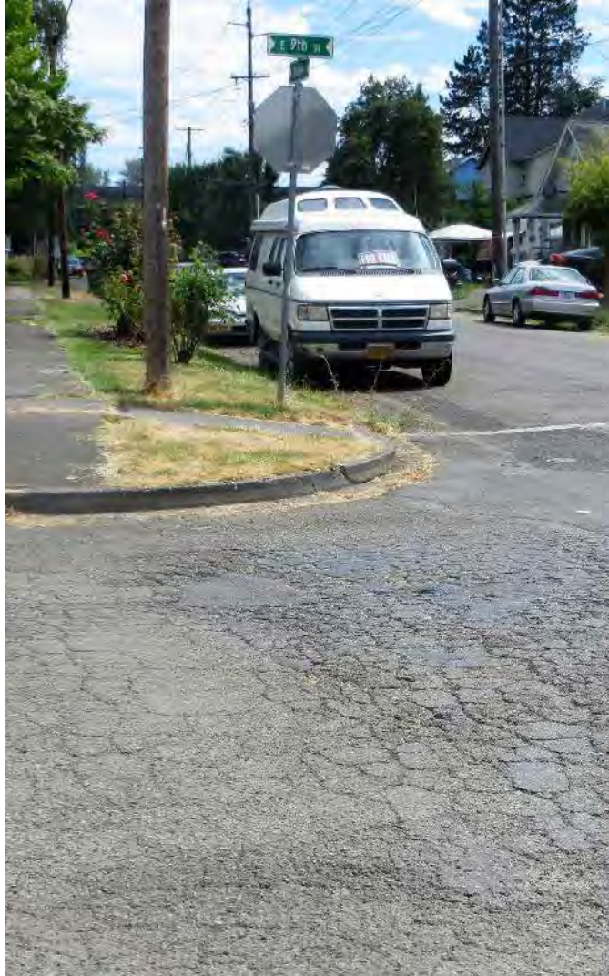
Poor roadway conditions along majority of routes: Cracks + Potholes (above)
