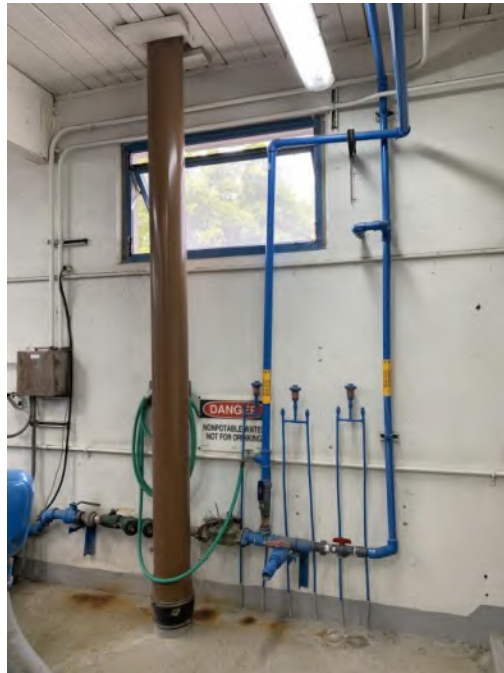
Figure 3.67 – Air Relief Piping Penetrating Laterally Unrestrained
