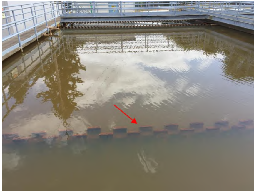
Figure 3.51 – Wooden Baffles in Sedimentation Basin No. 1
