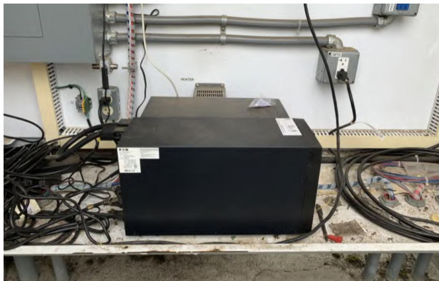
Figure 3.3 – Unrestrained Backup Batteries
