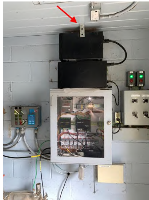
Figure 3.9 – Backup Batteries not Adequately Restrained
