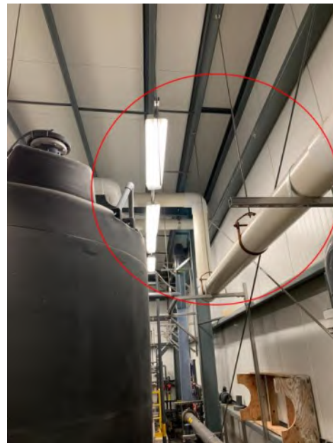
(b) Unbraced Piping Inside the Building
