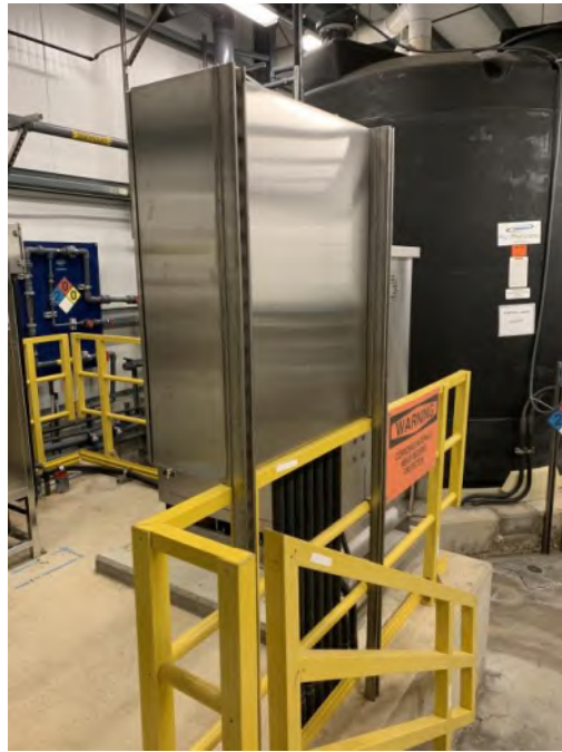
Figure 3.89 – Control Panel not Adequately Braced
