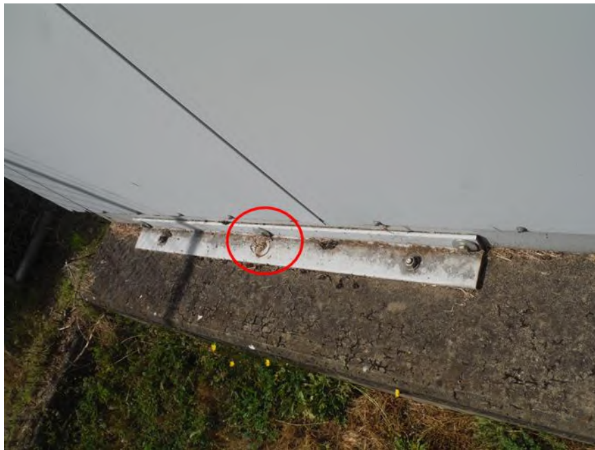
Figure 3.95 – Missing Anchors on Switchgear to Concrete Pad Connection
