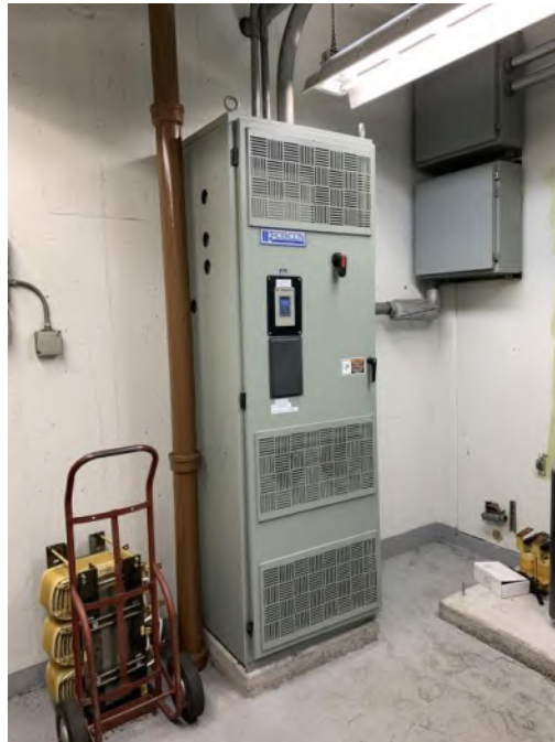
Figure 3.28 – Unbraced Cast Iron (Brittle) Vertical Pipe next to Electrical Cabinet
