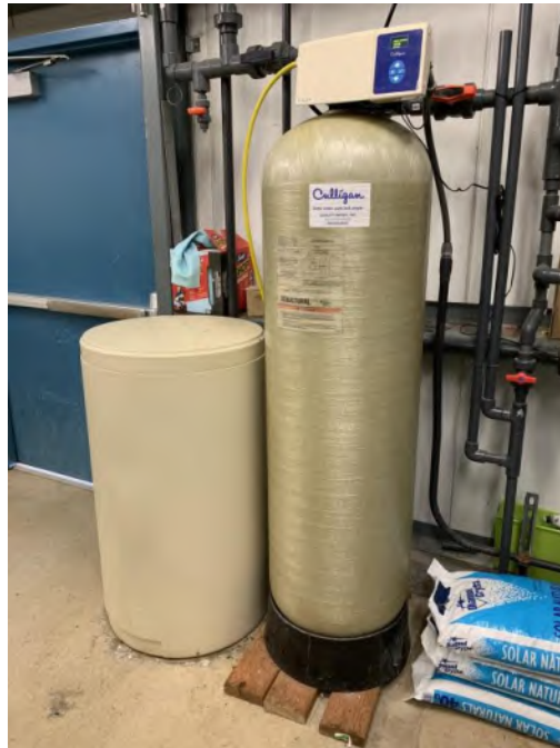
Figure 3.87 – Water Softener Components not Restrained
