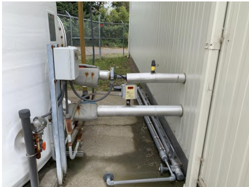
Figure 3.80 – Piping Connecting Salt Brine Tank to Sodium Hypochlorite Generation Building without Adequate Flexibility
