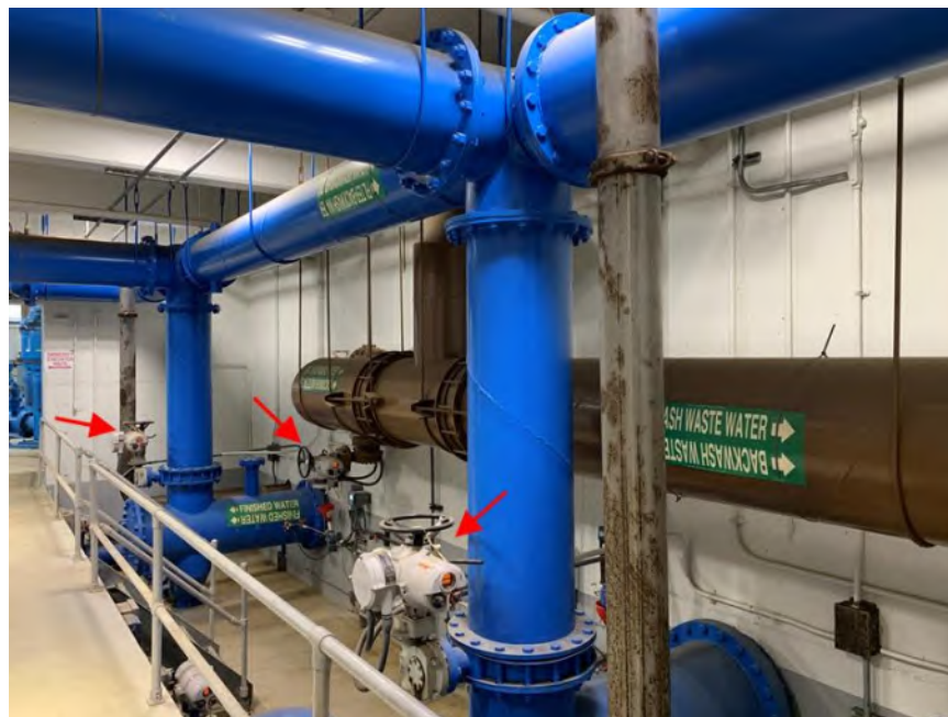
Figure 3.64 – Valves and Valve Actuators Installed In-Line with Piping Systems not Independently Braced
