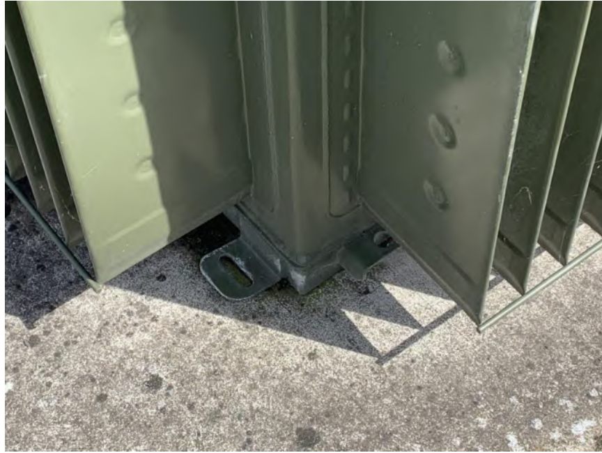
Figure 3.96 – Electrical Transformer not Anchored to Concrete Pad
