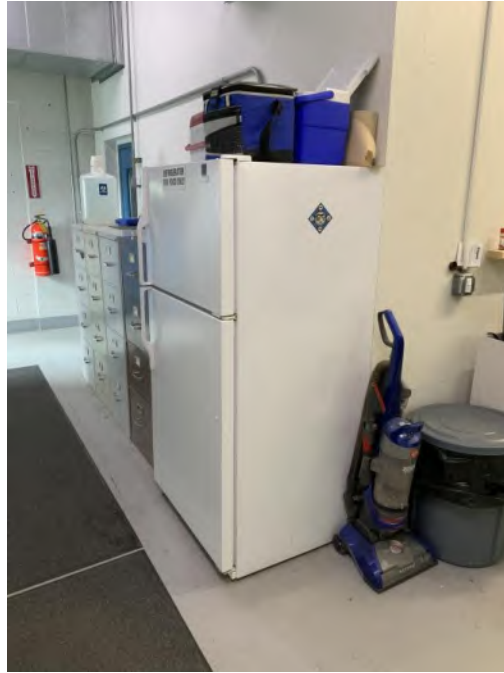
Figure 3.30 – Unrestrained Refrigerator and Filing Cabinets Adjacent to Walkway
