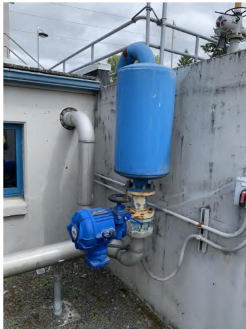
Figure 3.66 – Air Vent Valve and Muffler not Adequately Braced
