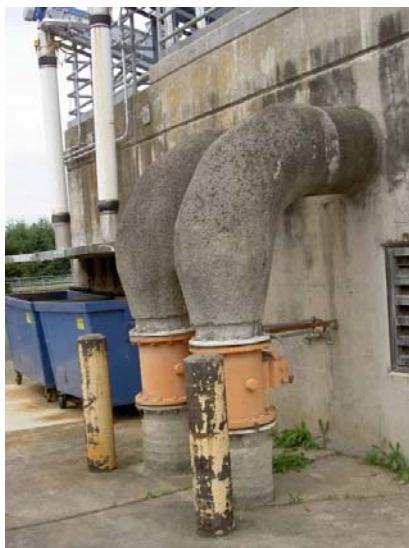
Figure 3-4. Influent Flowmeters at the WWTP Headworks
