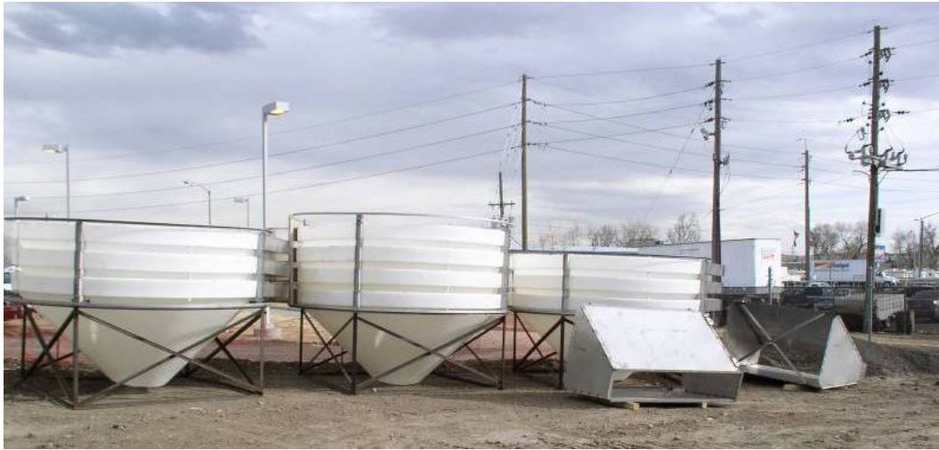
Figure ES-9. Photo of Gravity Plate Type Settler for Grit Removal
