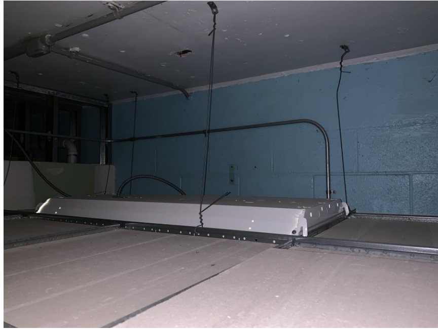
Figure 3.46 – Light Fixture Supported by Ceiling Grid
