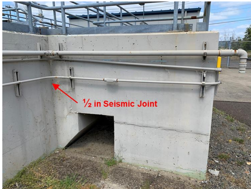
Figure 3.50 – Sedimentation Basins Effluent Structure (Outlet Basin Structure)
