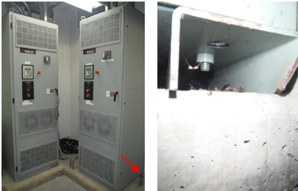
Figure 3.27 – Electrical Cabinets with Missing Anchor at the Base
