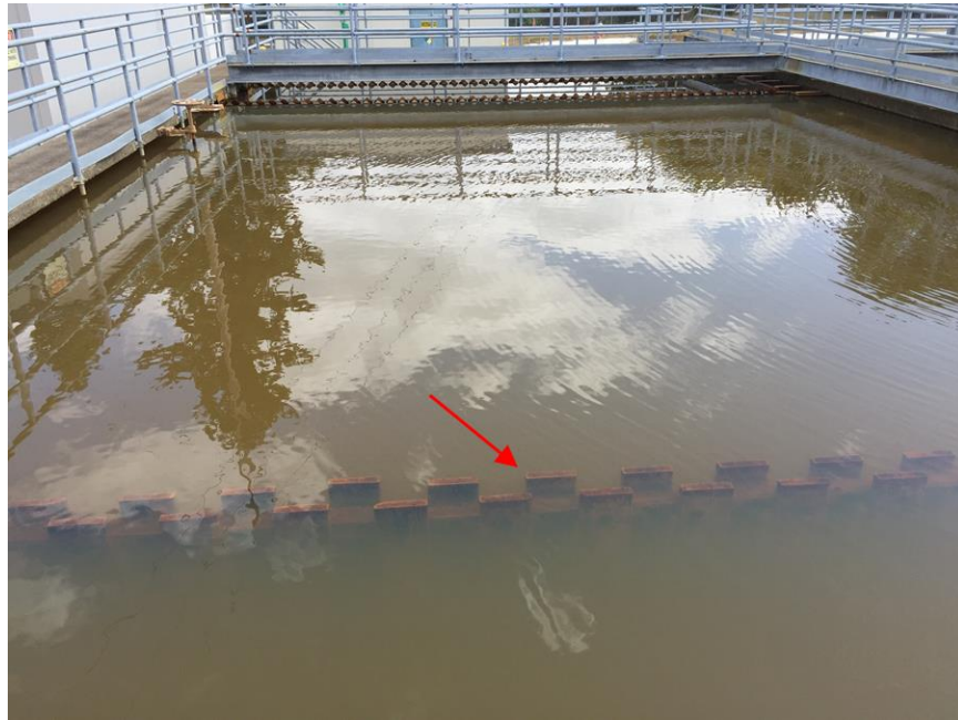
Figure 3.51 – Wooden Baffles in Sedimentation Basin No. 1
