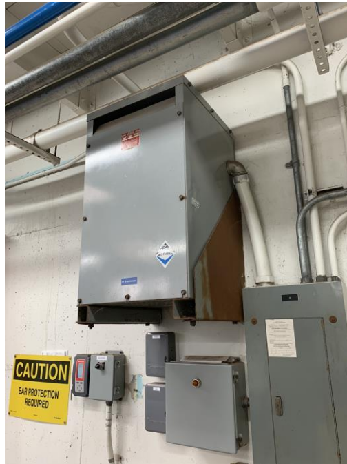
Figure 3.69 – Electrical Transformer not Adequately Braced Against Movement Parallel to Wall
