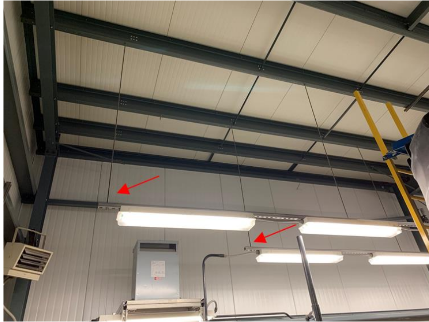
Figure 3.91 – Unrestrained Light Fixtures
