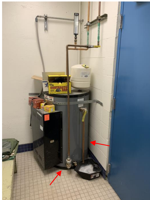
Figure 3.45 – Water Heater Tank not Adequately Restrained
