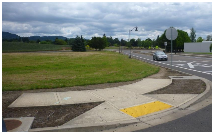
ADA Compliant Curb Ramp with No Connections
