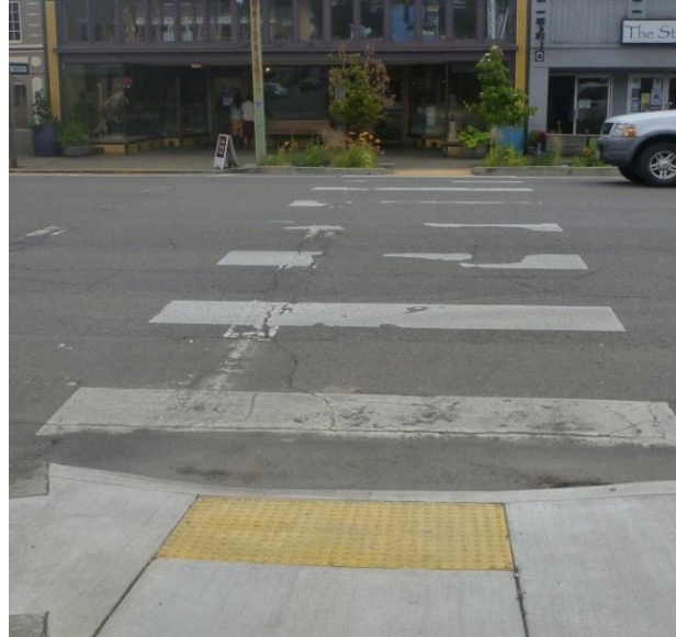
Faded Crosswalk in Downtown Newberg
