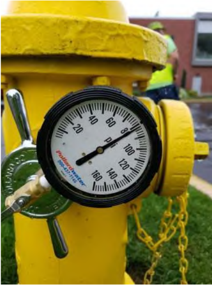
Residual pressure on flowed hydrant at intersection of Fulton Street and East Cherry Street
