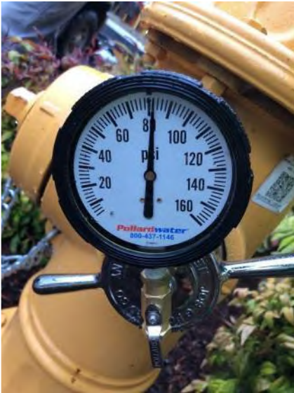
Residual Pressure on guage hydrant in front of 1013 N Center Street
