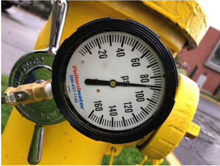
Static pressure on flowed hydrant at intersection of Fulton Street and East Cherry Street
