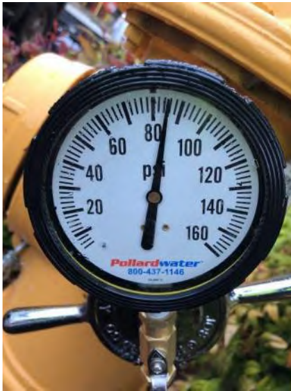
Static pressure on gauge hydrant located in front of 1013 N Center Street.
