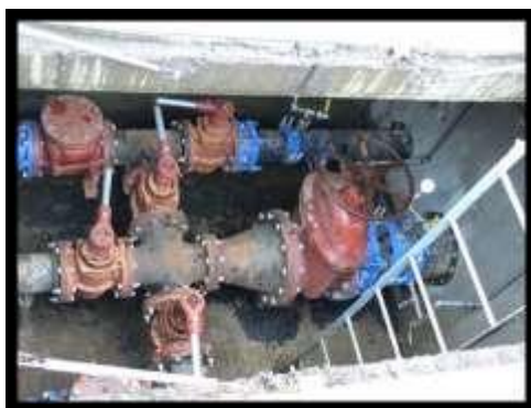
FIGURE 24 FERNWOOD VALVE VAULT
