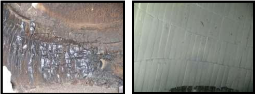
FIGURE 12 DEHYDRATION UNIT BURNER BEFORE AND AFTER CONDITION
