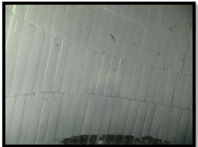
FIGURE 6 DEHYDRATION UNIT BURNER BEFORE AND AFTER CONDITION
