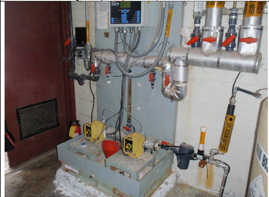
Photo 2 – Metering Pumps (System replaced in Summer 2017)
