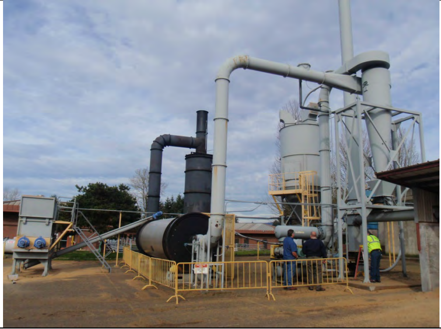
Photo 1 – Sawdust Dryer System
