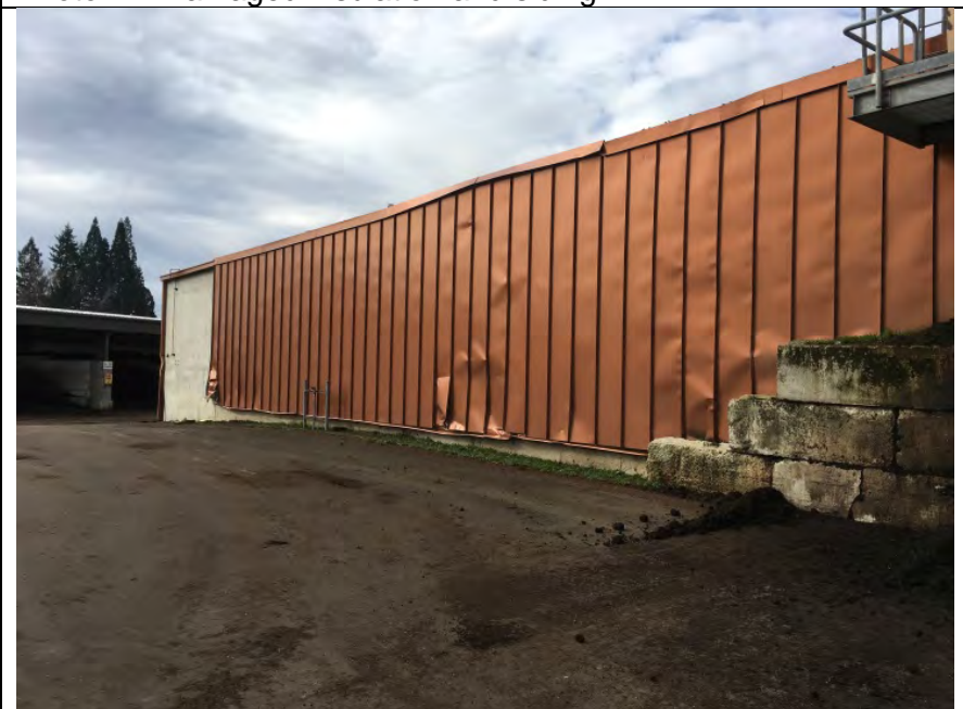
Photo 7 – Damaged insulation and siding
