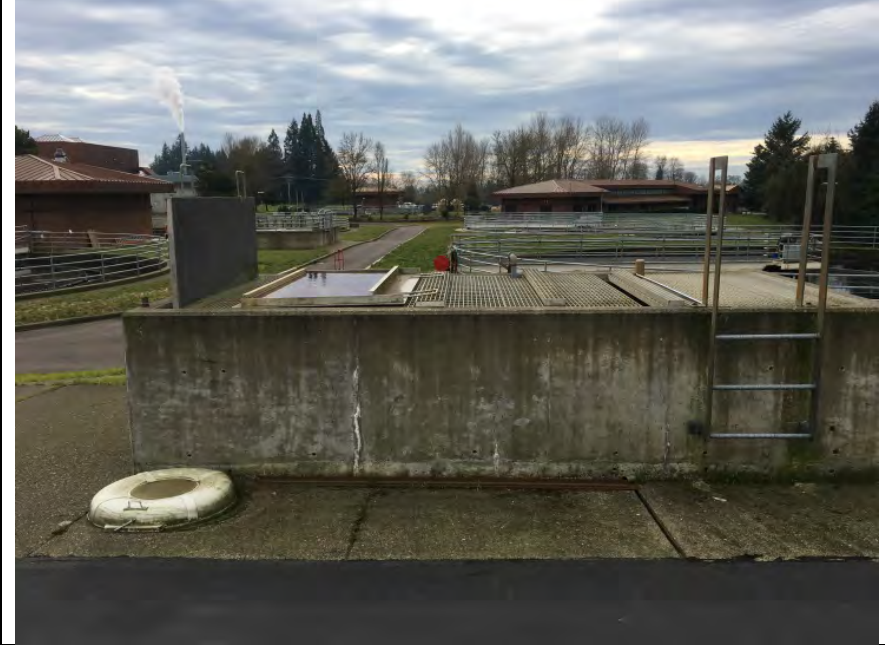
Photo 2 – RDS Distribution Box (northeast side)
