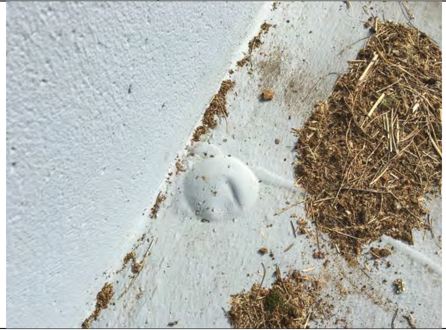
Photo 3 – Floor Coating Bubbles
