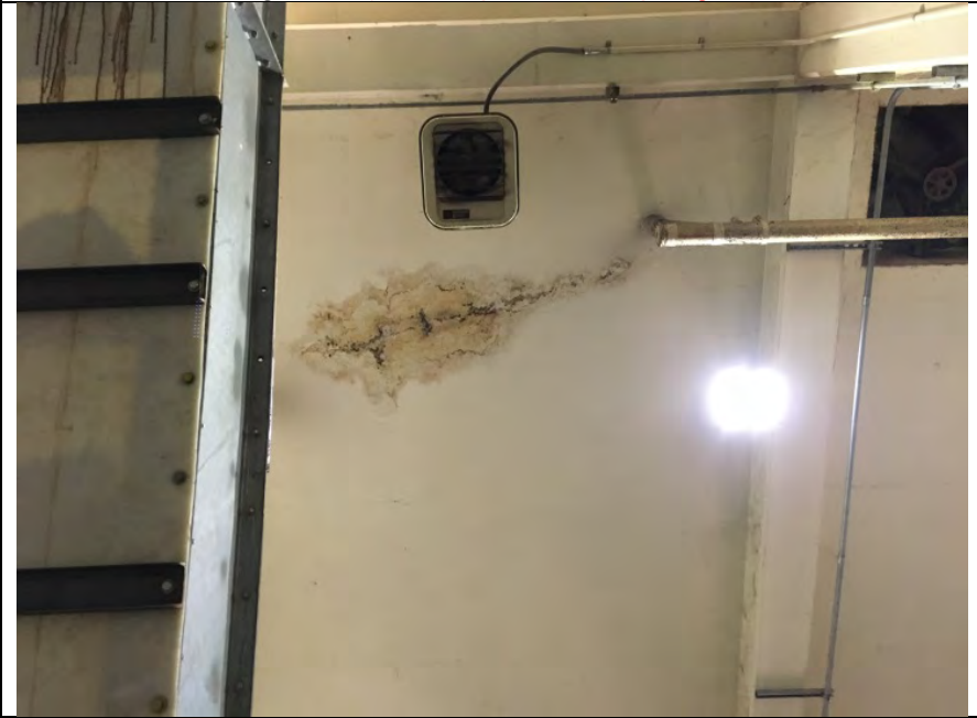
Photo 4 – Leaking Roof (Roof replaced in Spring 2017)
