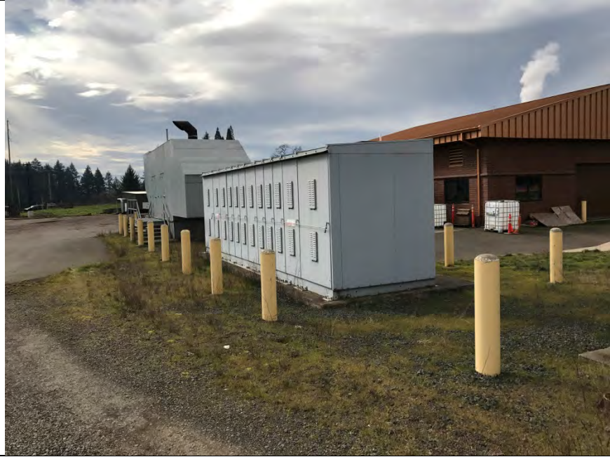
Photo 1 – Switchgear and Generator
