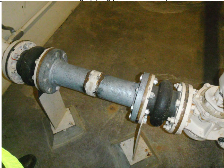
Photo 4 – WAS discharge piping potential failure point
