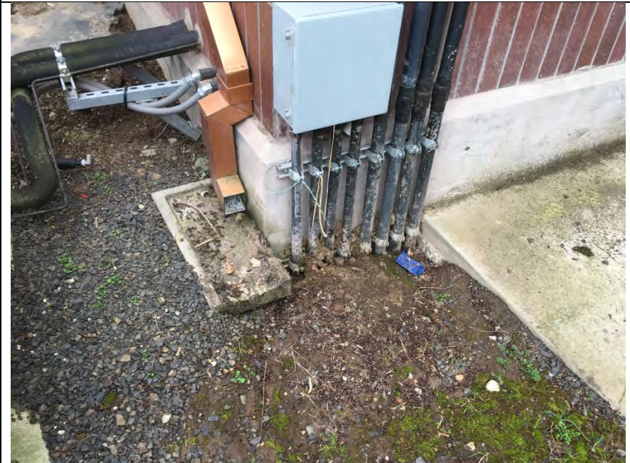
Photo 2 – Gutter splashing causing erosion around electrical conduits
