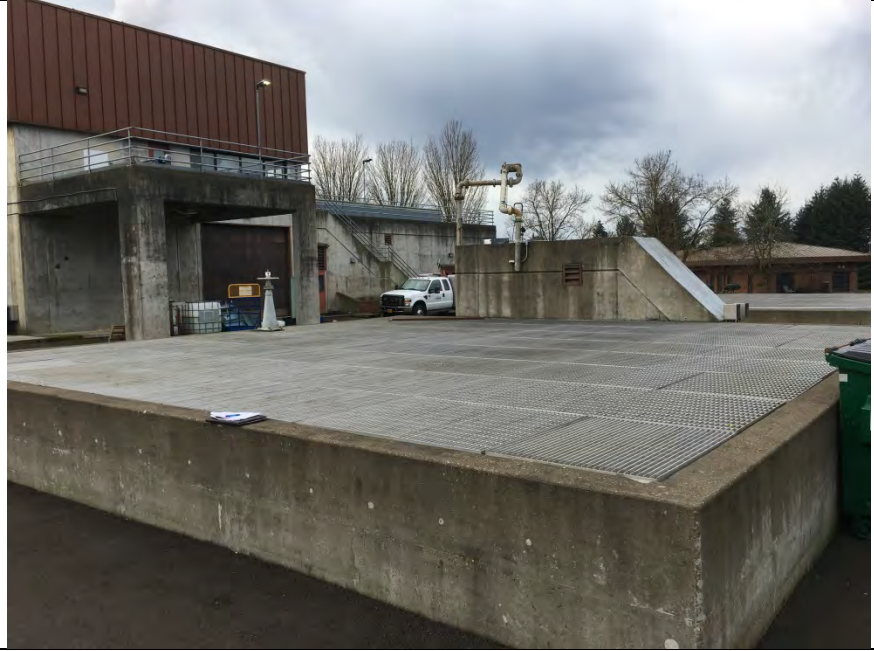
Photo 1 – Sludge Storage Tanks
