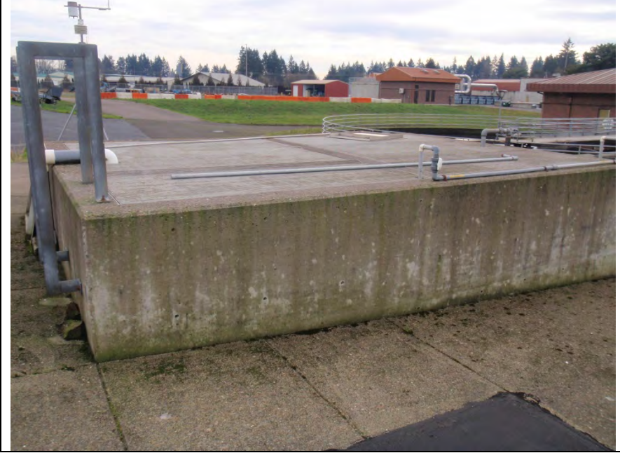
Photo 1 – RDS Distribution Box (northwest side)
