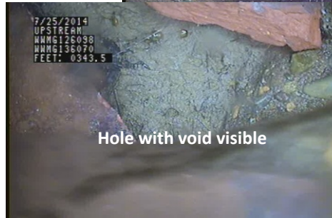
Offset, cracked lateral blocked with dirt
