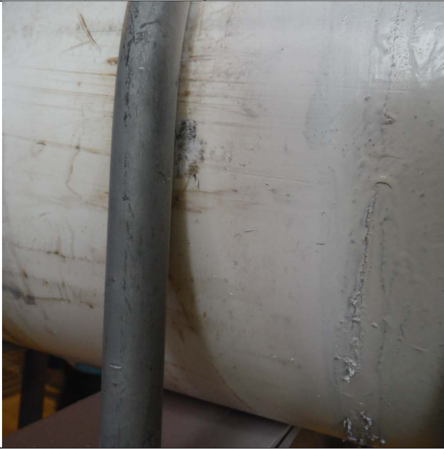
Photo 3 – Pipe support rubbing
