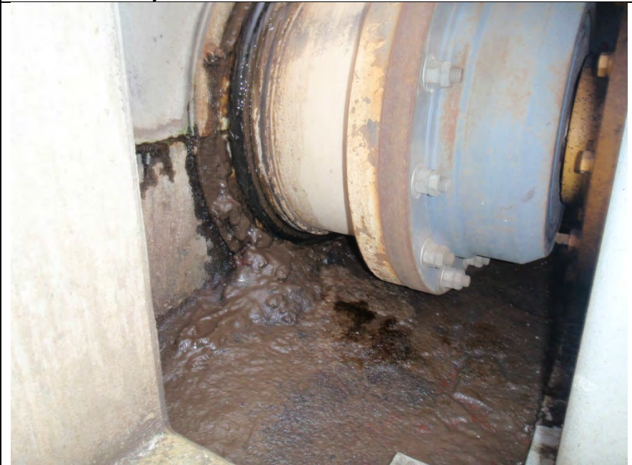
Photo 2 – Leaky Rotor Seal
