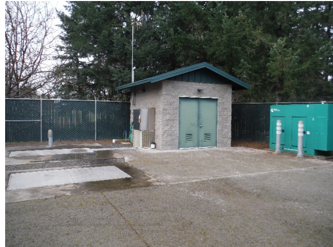
Highway 240 Lift Station
