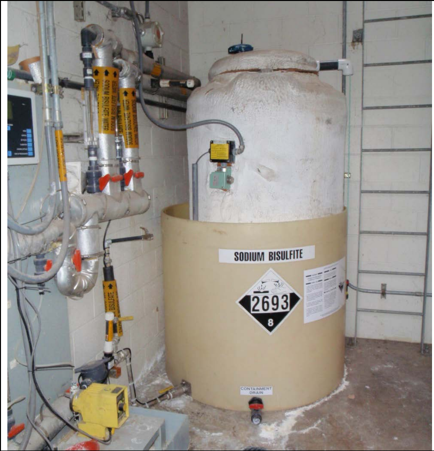
Photo 1 – Sodium Bisulfite System (System replaced in Summer 2017)
