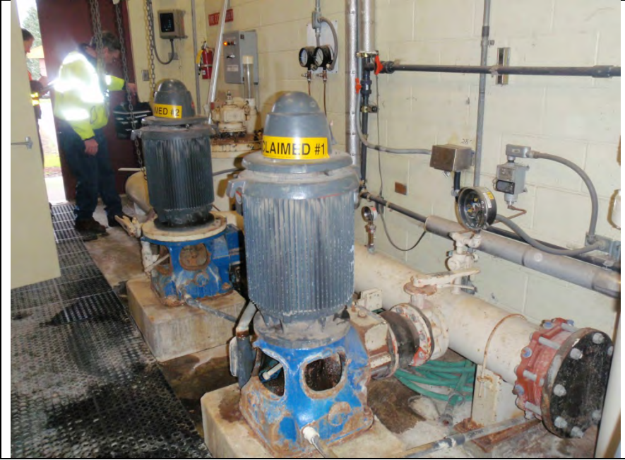
Photo 1 – Reclaimed Water Pumps
