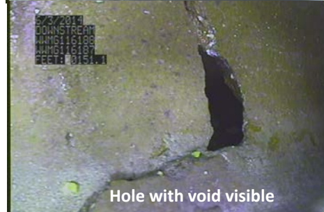
Holes and surface damage
