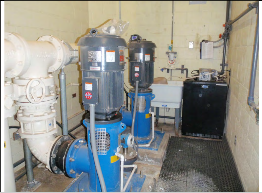
Photo 3 – Reuse Water Pumps
