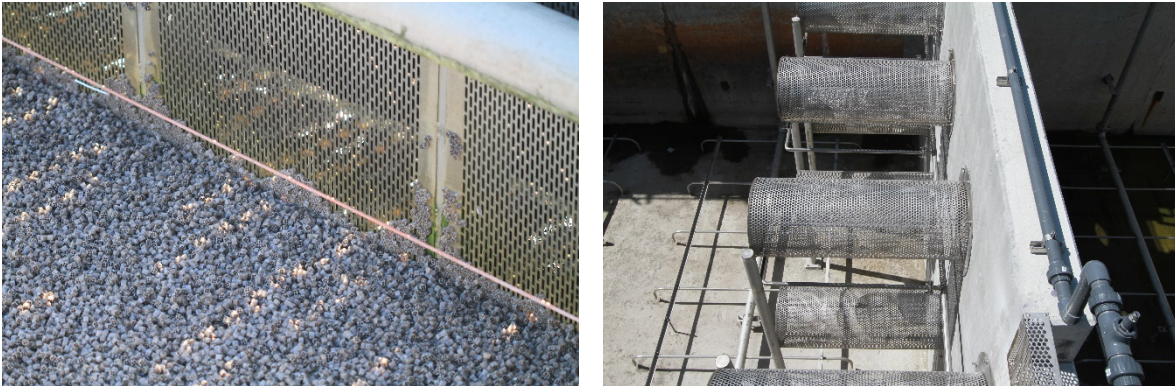
Figure 10-9: MBBR Screen Photos
