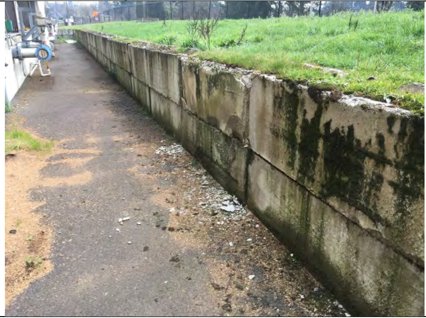
Photo 3 – Retaining wall deterioration
