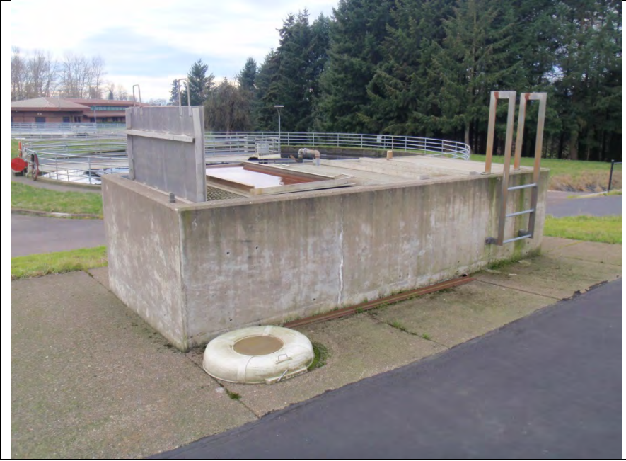
Photo 1 – RAS Distribution Box
