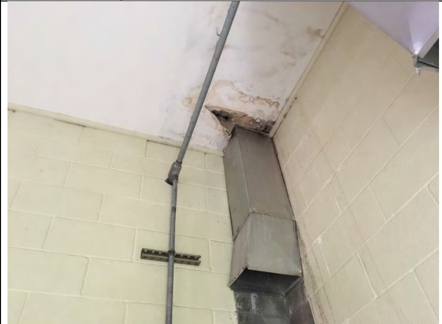
Photo 2 – Water Damage (water damaged sheetrock was replaced in Spring 2017)
