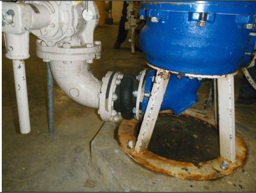
Photo 3 – WAS Pump 3 inlet piping misalignment and poor pipe support
