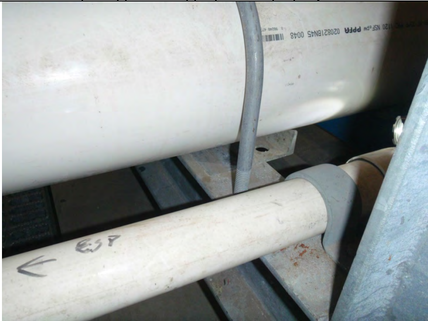
Photo 4 – Pipe support not appropriate or properly installed
