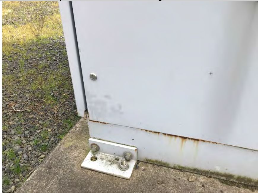
Photo 2 – Sample of corrosion on switchgear
