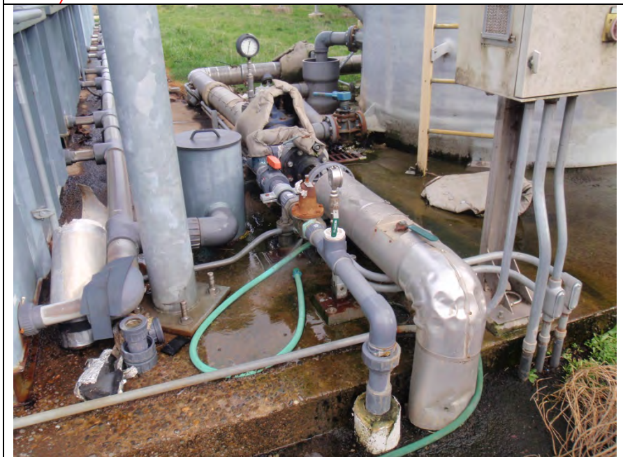
Photo 3 – Piping (Water piping improvements made in Summer 2017)
