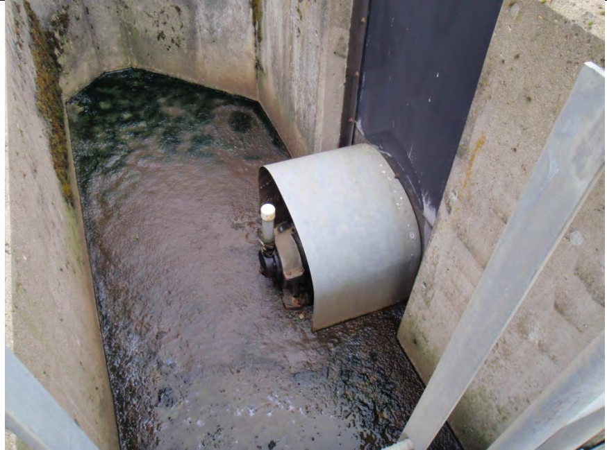
Photo 2 – Leaky Rotor Seal
