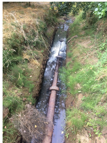
Exposed Hess Creek Pipeline
