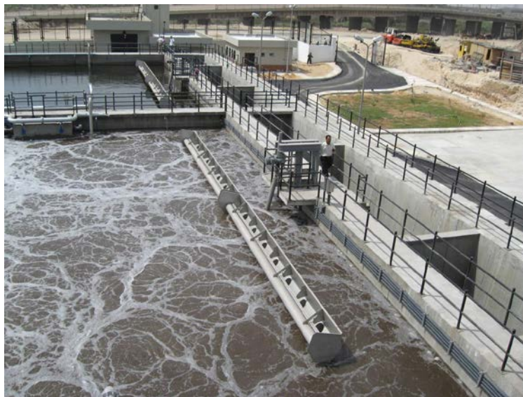
Figure 10-7: Example of SBR Installation
