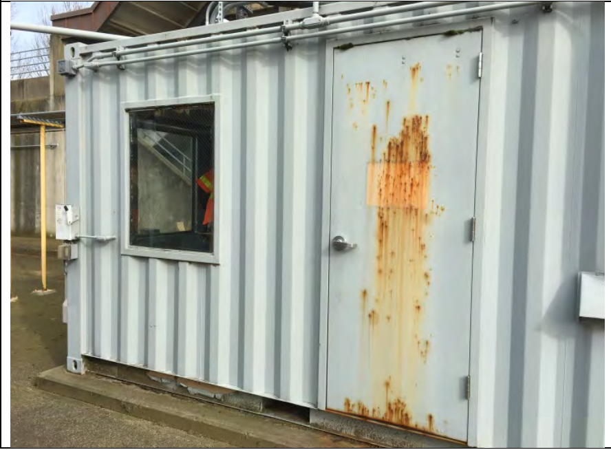
Photo 3 – MCC Container Corrosion
