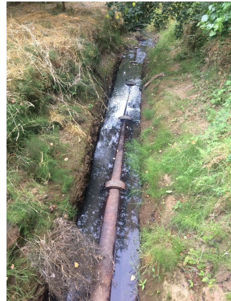
Exposed Hess Creek Pipeline
