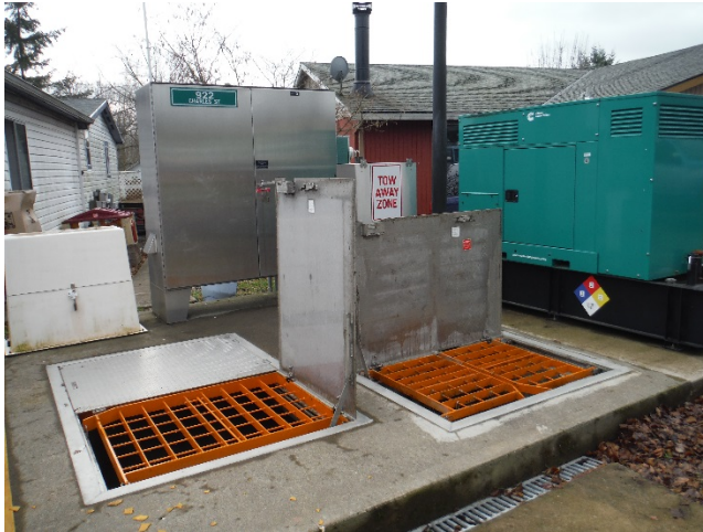
Charles Lift Station
