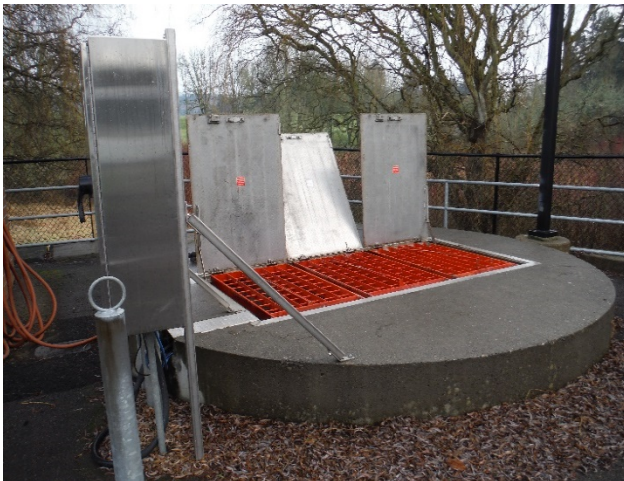
Fernwood Lift Station
