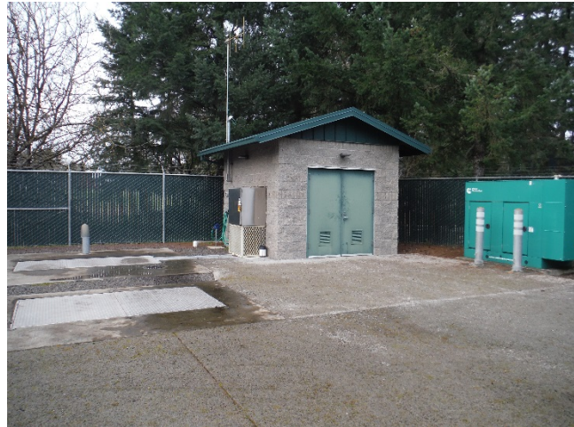
Highway 240 Lift Station
