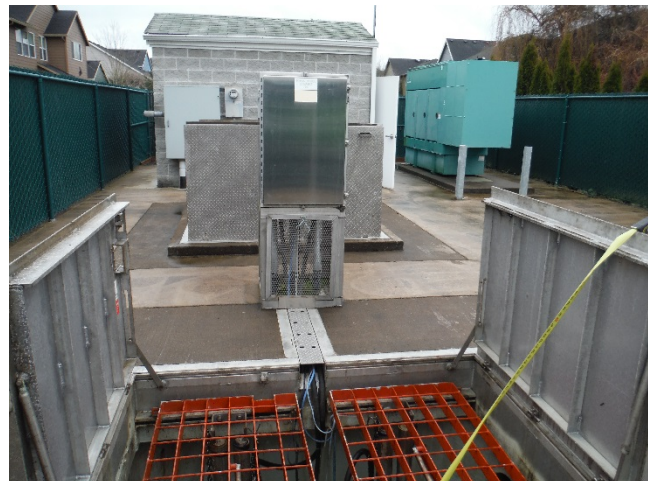
Chehalem Lift Station
