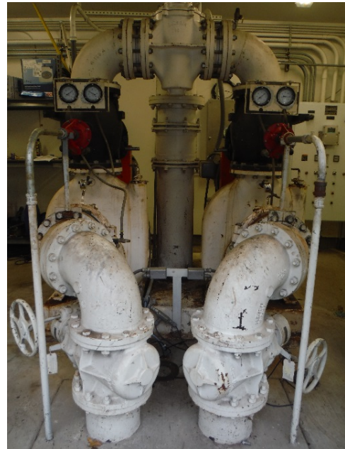
Dayton Lift Station
