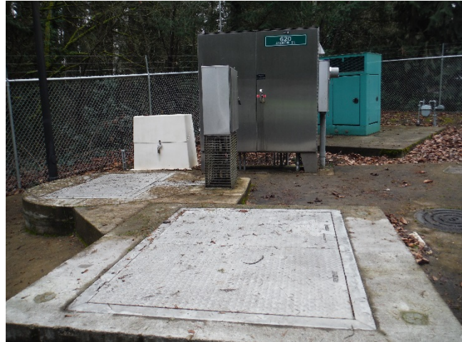
Andrew Lift Station
