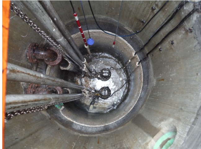
Creekside Lift Station
