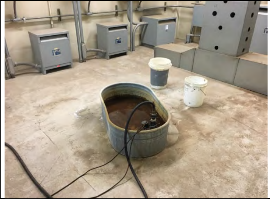
Photo 6 – Collection of water from roof leak (Roof replaced in Spring 2017)
