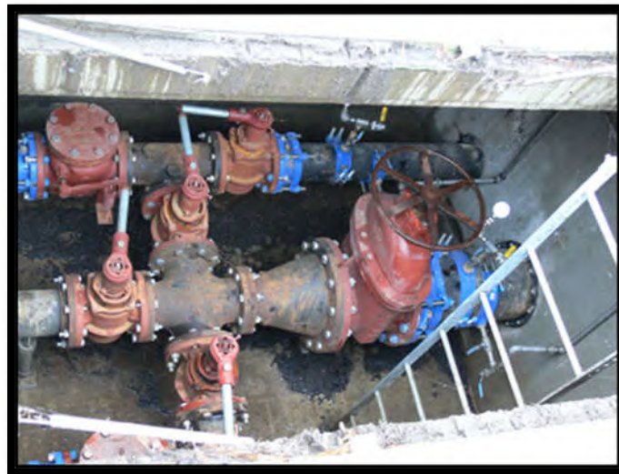
FIGURE 16 FERNWOOD VALVE VAULT
