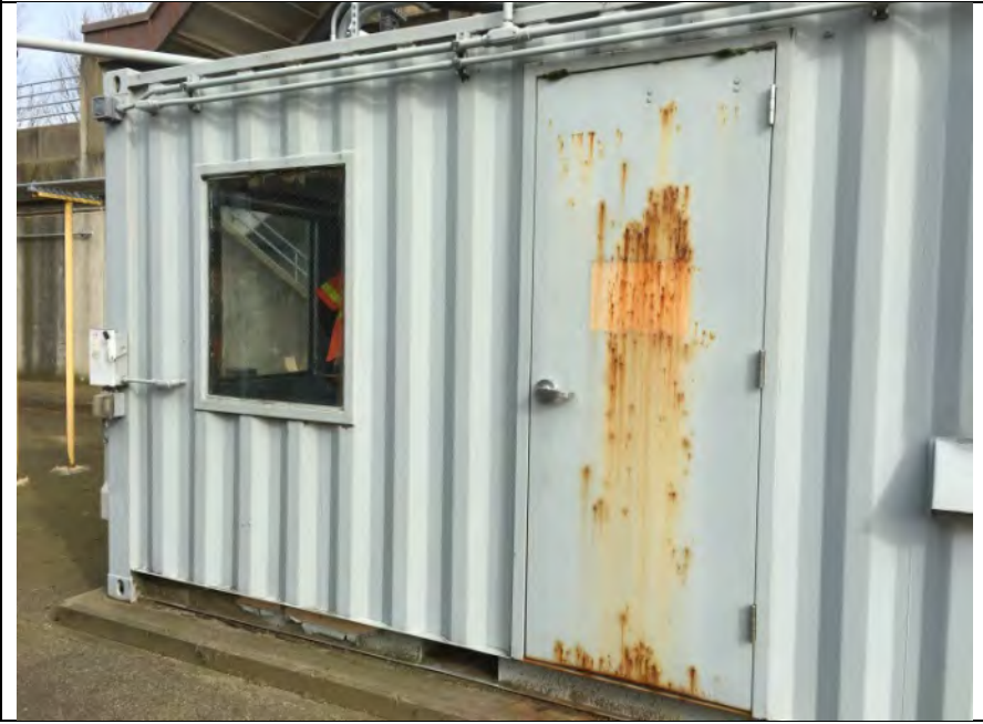
Photo 3 – MCC Container Corrosion
