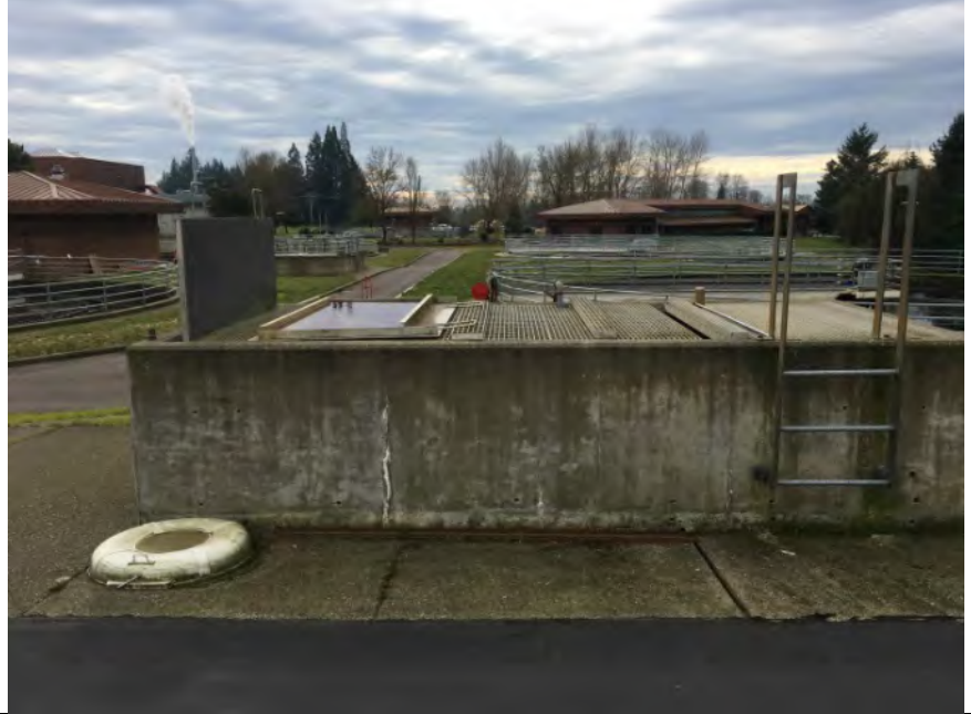
Photo 2 – RDS Distribution Box (northeast side)
