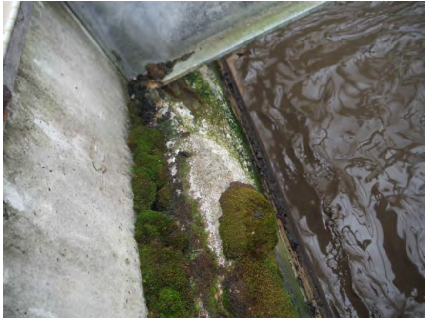
Photo 2 – Portion of concrete missing and buildup of moss
