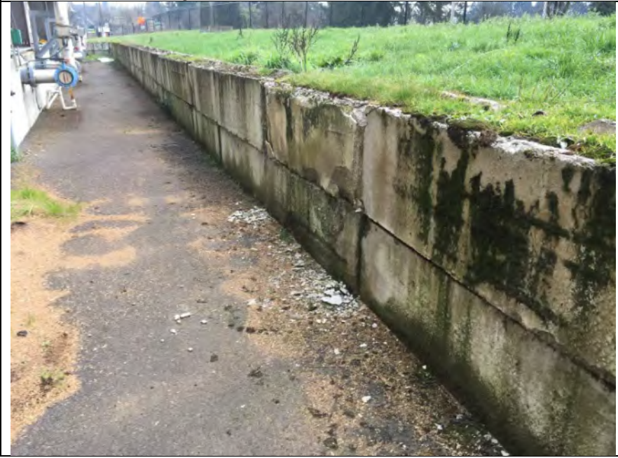
Photo 3 – Retaining wall deterioration
