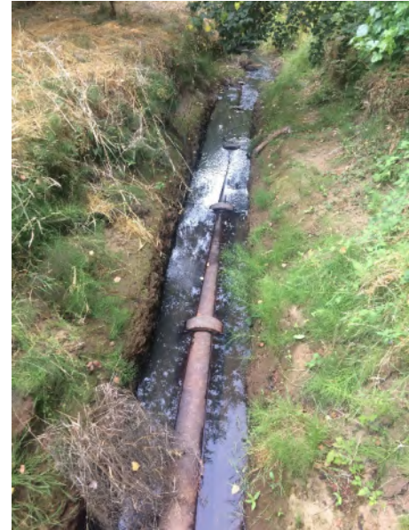
Exposed Hess Creek Pipeline
