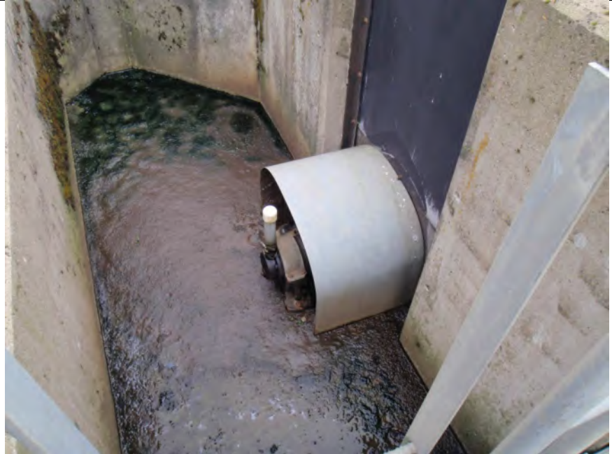
Photo 2 – Leaky Rotor Seal
