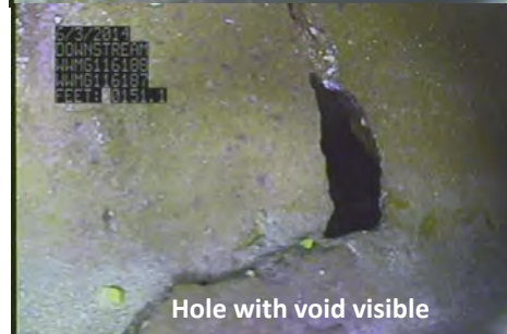
Holes and surface damage
