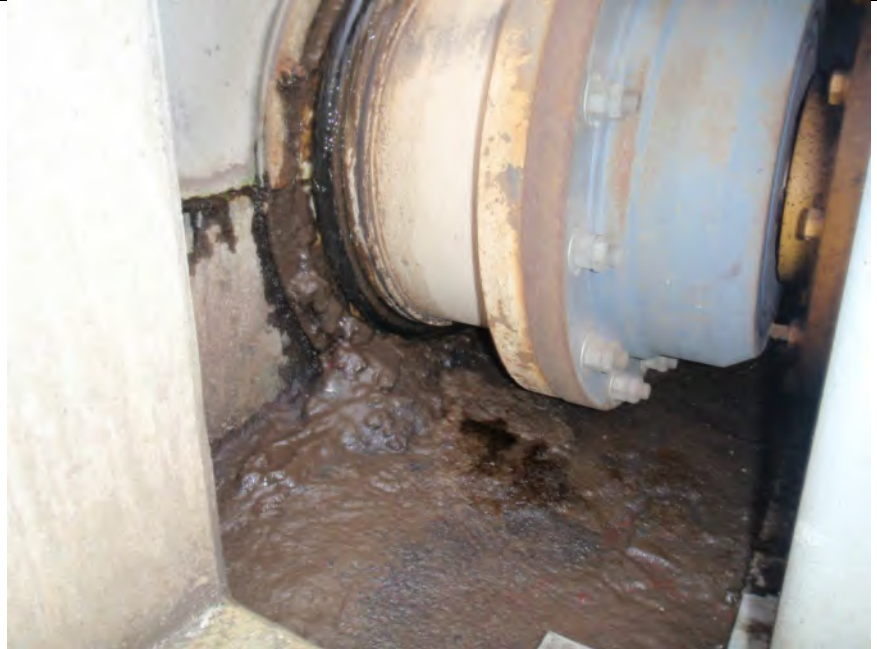
Photo 2 – Leaky Rotor Seal
