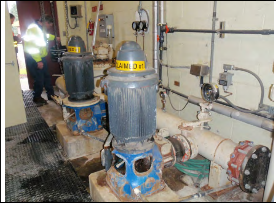
Photo 1 – Reclaimed Water Pumps
