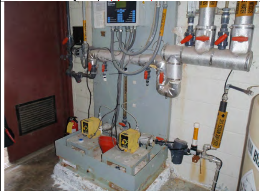
Photo 2 – Metering Pumps (System replaced in Summer 2017)
