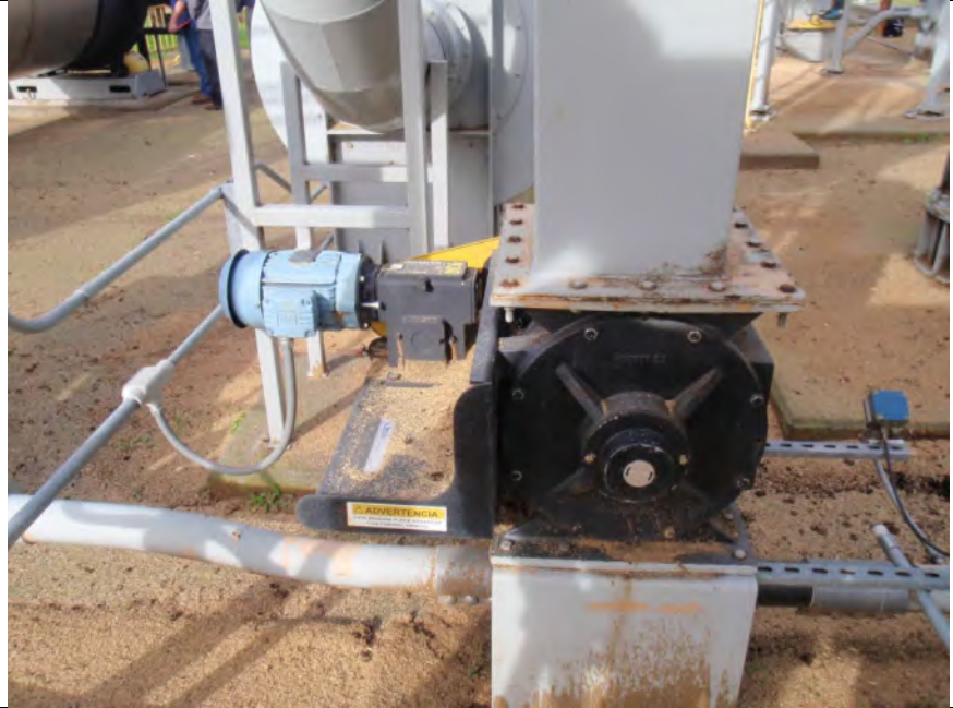
Photo 2 – Lower Air Lock (Air Lock replaced in Summer 2017)
