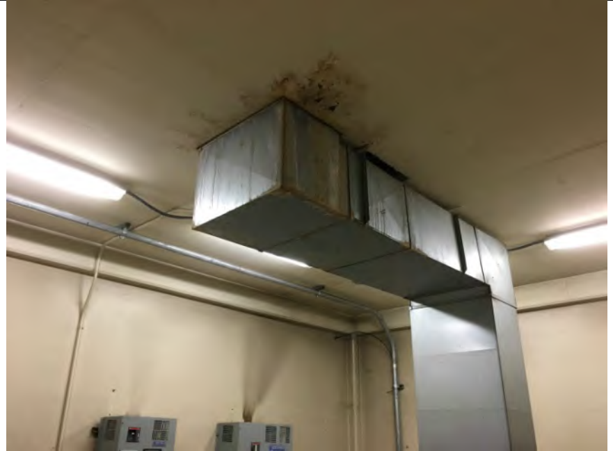
Photo 5 – Leak around HVAC duct (Roof replaced in Spring 2017)
