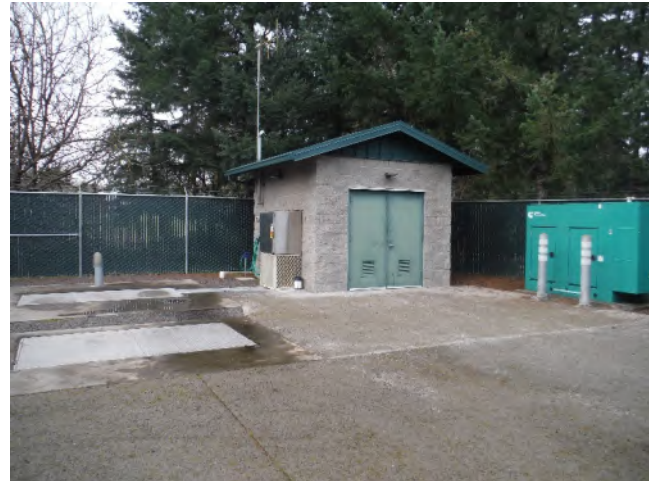
Highway 240 Lift Station
