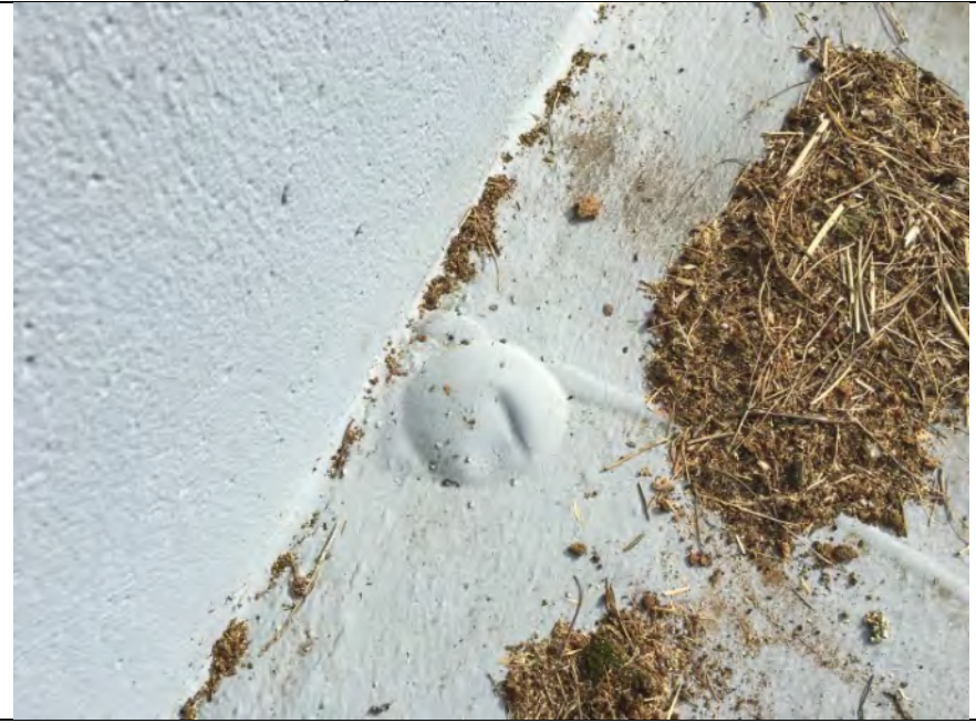
Photo 3 – Floor Coating Bubbles
