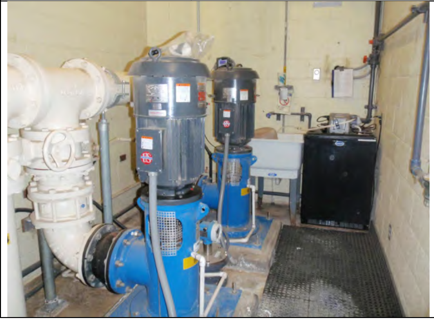
Photo 3 – Reuse Water Pumps
