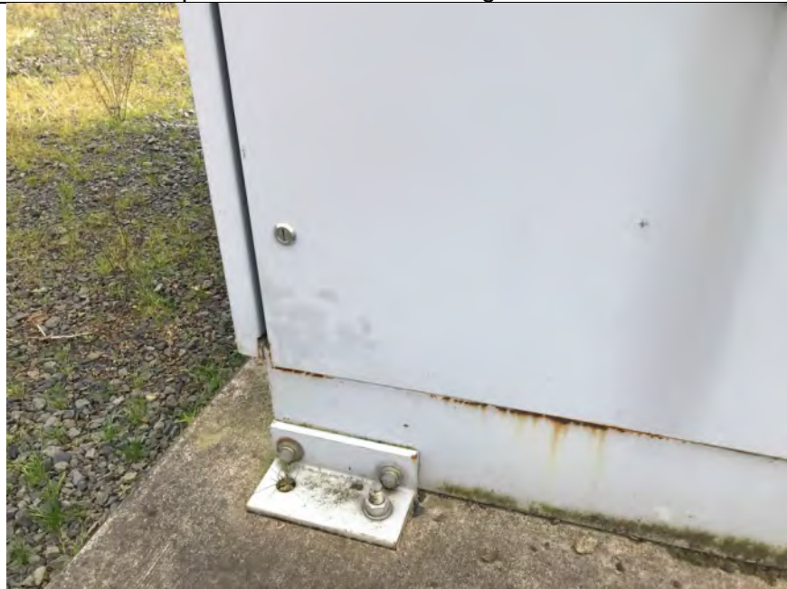
Photo 2 – Sample of corrosion on switchgear
