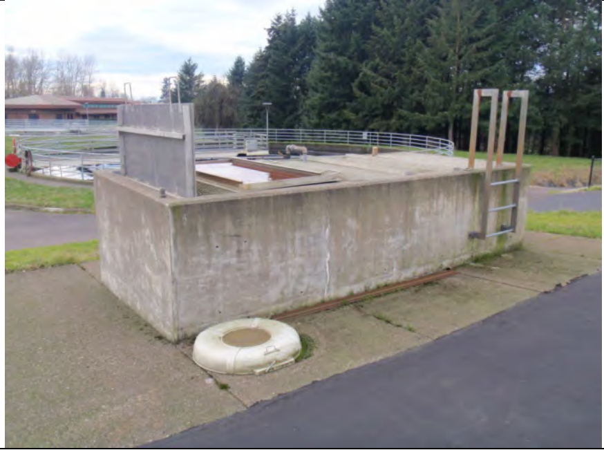
Photo 1 – RAS Distribution Box
