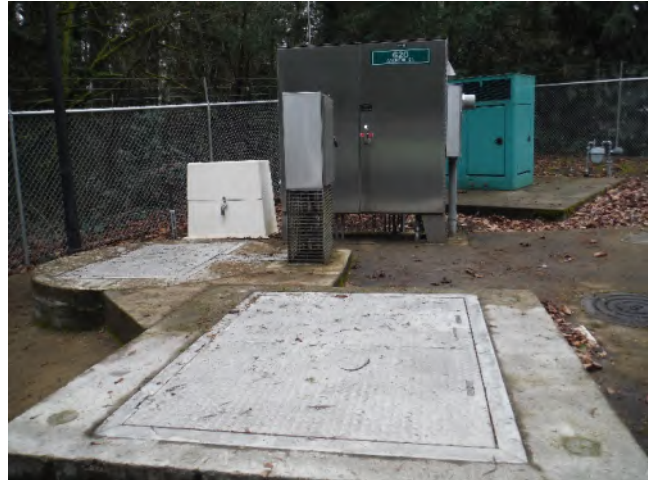
Andrew Lift Station
