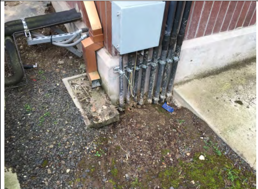
Photo 2 – Gutter splashing causing erosion around electrical conduits
