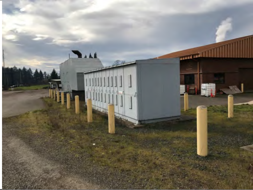
Photo 1 – Switchgear and Generator
