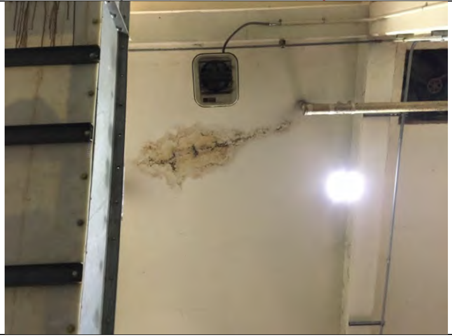
Photo 4 – Leaking Roof (Roof replaced in Spring 2017)
