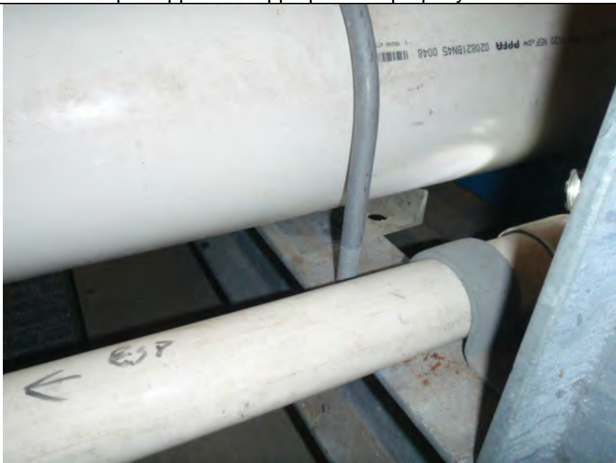
Photo 4 – Pipe support not appropriate or properly installed
