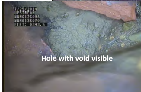
Offset, cracked lateral blocked with dirt
