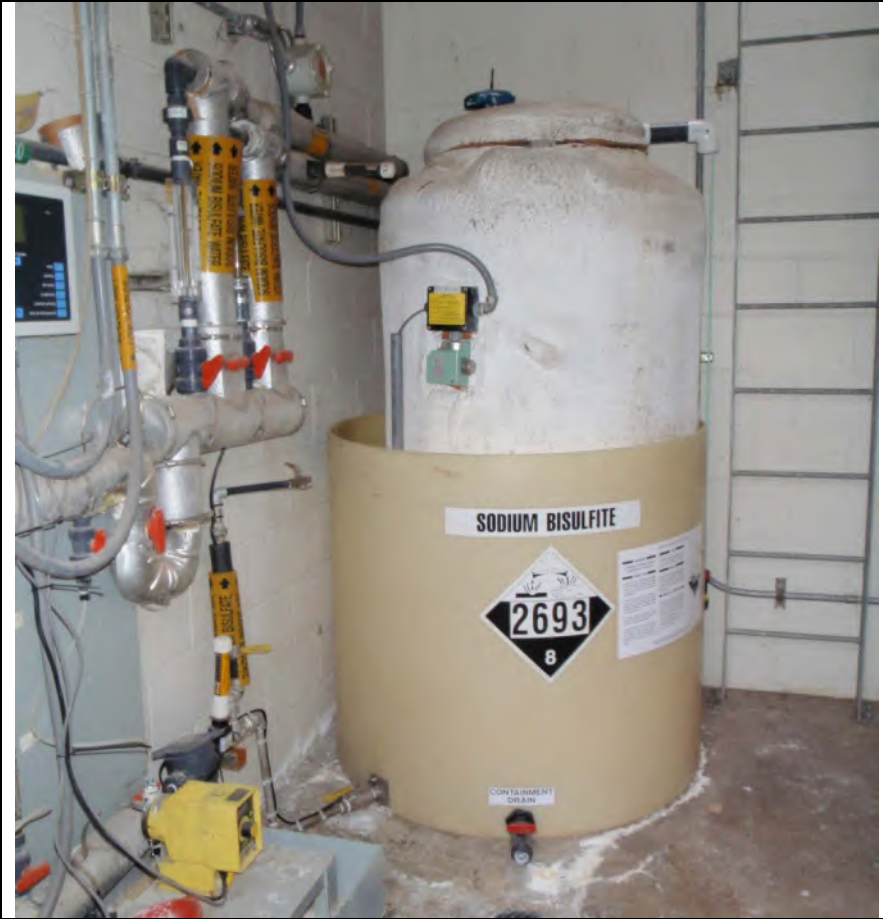
Photo 1 – Sodium Bisulfite System (System replaced in Summer 2017)
