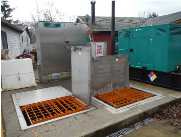
Charles Lift Station
