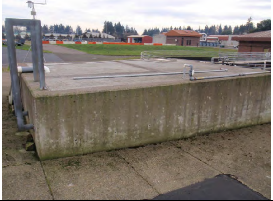
Photo 1 – RDS Distribution Box (northwest side)
