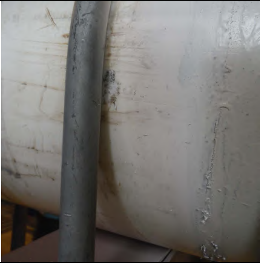
Photo 3 – Pipe support rubbing
