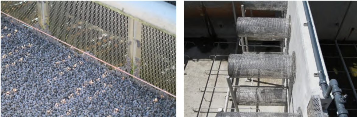
Figure 10-9: MBBR Screen Photos
