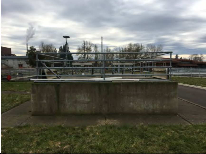
Photo 1 – Clarifier Distribution Box
