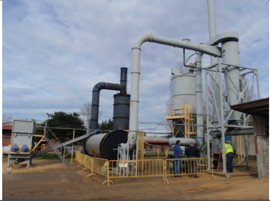
Photo 1 – Sawdust Dryer System
