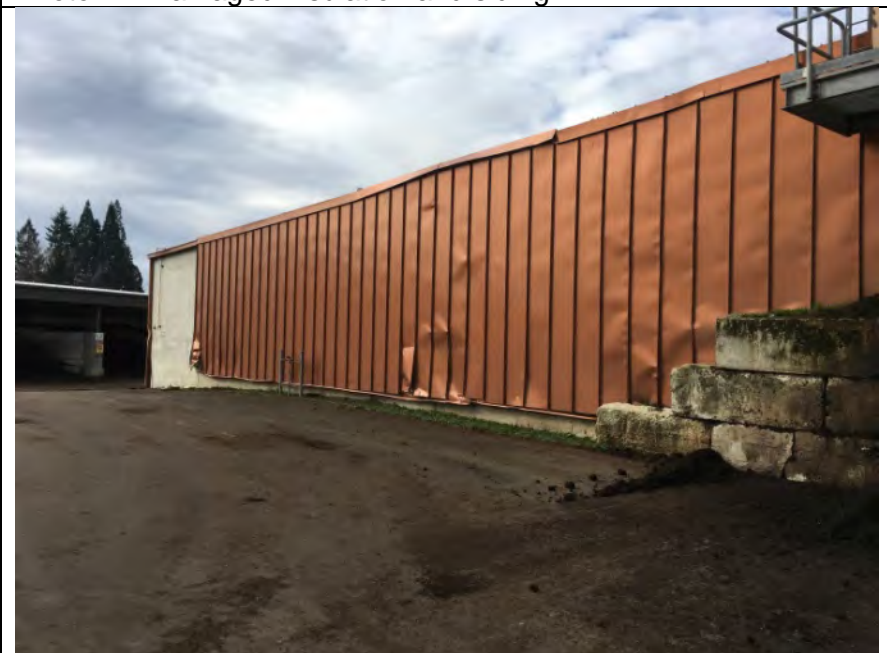
Photo 7 – Damaged insulation and siding
