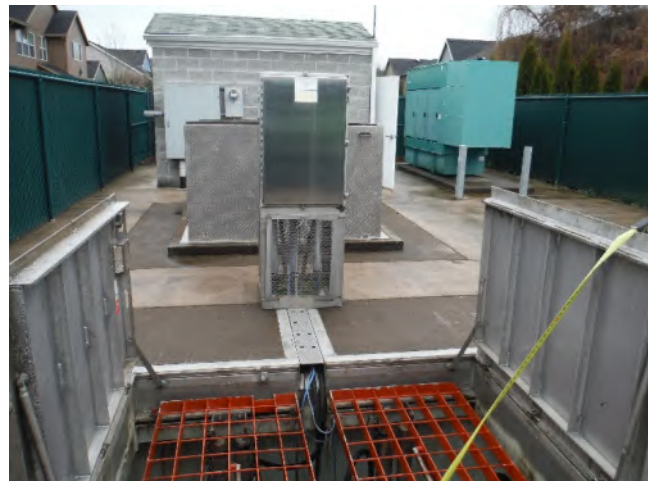
Chehalem Lift Station
