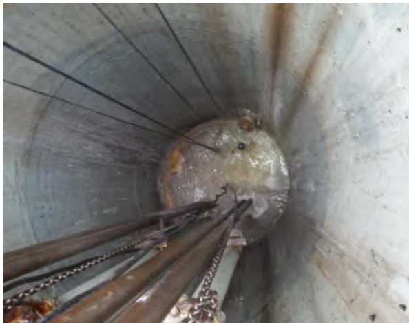
Sheridan Lift Station
