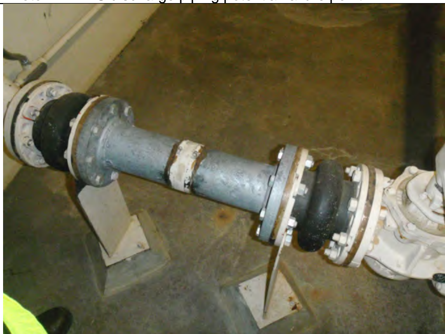
Photo 4 – WAS discharge piping potential failure point
