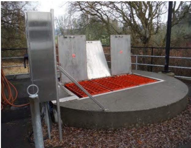
Fernwood Lift Station
