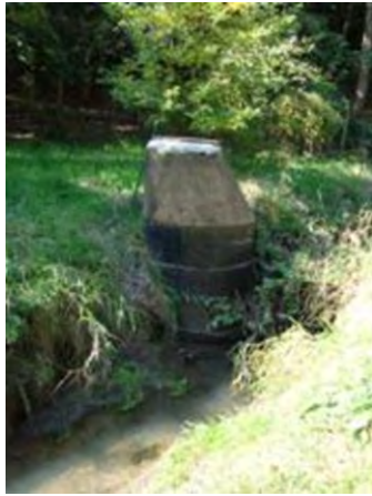
Example photos of stream reach above Crestview. Significant bank erosion in this reach.
