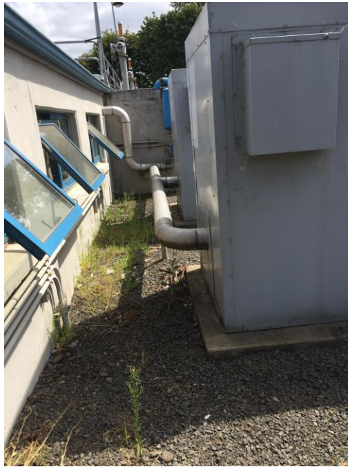
Figure 3.65 – Air Scour Piping from Blowers to Filter Gallery without Adequate Flexibility to Accommodate Differential Movement
