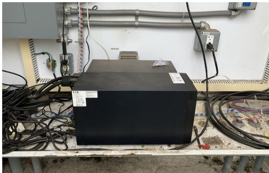
Figure 3.3 – Unrestrained Backup Batteries
