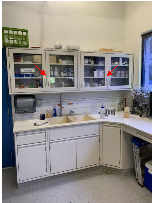
Figure 3.44 – Chemical Cabinet Doors without Proper Latches
