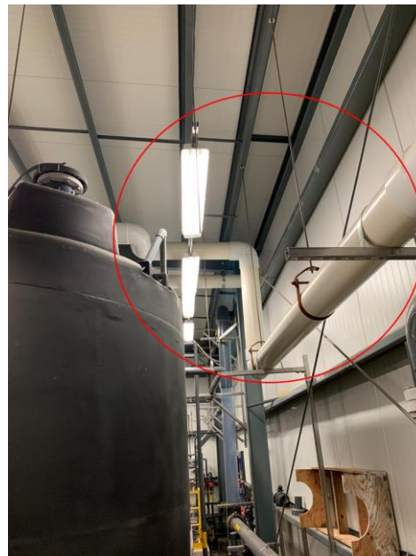
(b) Unbraced Piping Inside the Building
