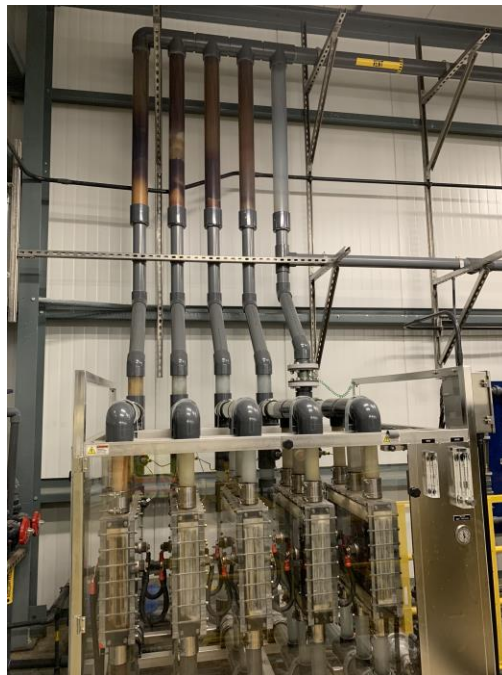
Figure 3.84 – Lack of Flexibility in Piping between Sodium Hypochlorite Generator and Attachment to Building
