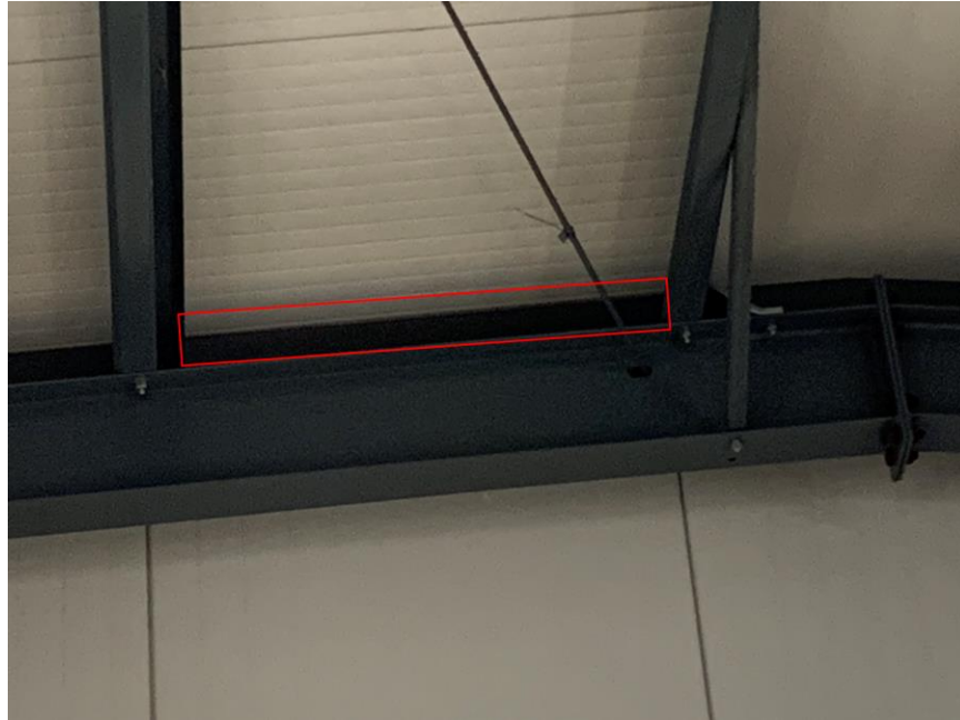
Figure 3.75 – Inadequate Load Path from Roof Diaphragm to Moment Frame Beams (no Blocking between Purlins)
