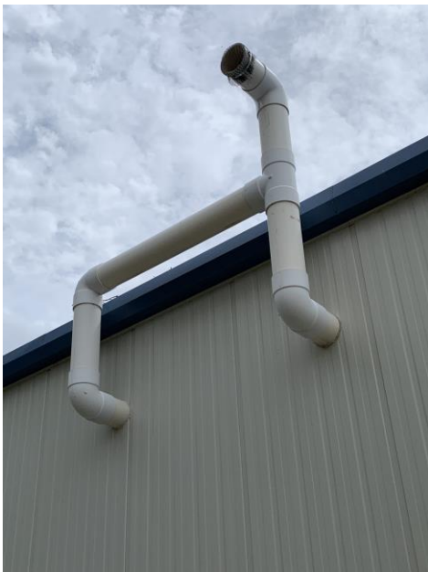
(a) Unbraced Piping Outside the Building
