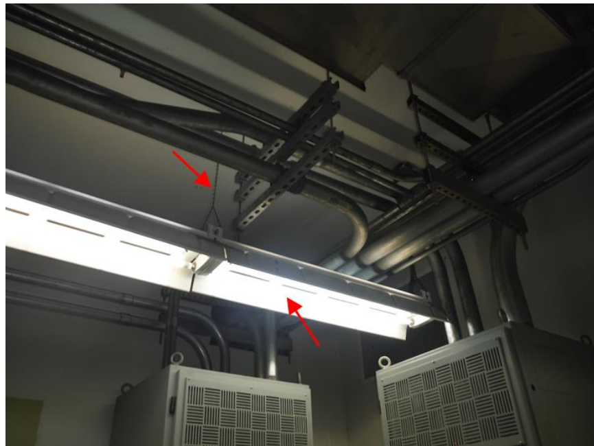
Figure 3.29 – Lights on Pendant Supports not Restrained and without Lens Covers
