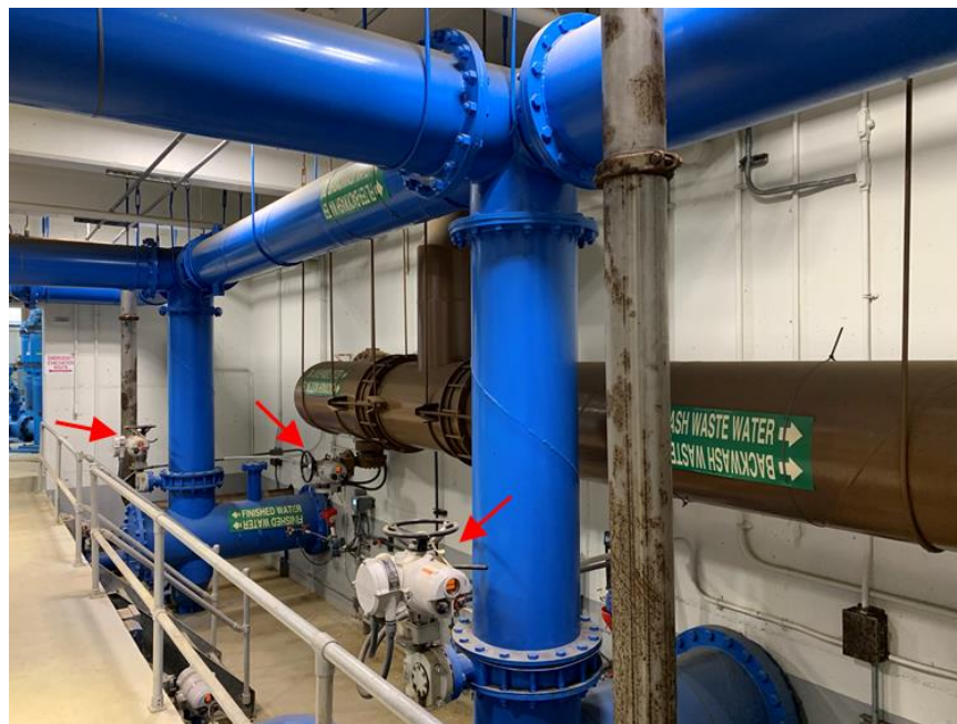
Figure 3.64 – Valves and Valve Actuators Installed In-Line with Piping Systems not Independently Braced
