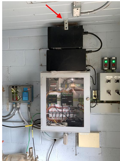
Figure 3.9 – Backup Batteries not Adequately Restrained
