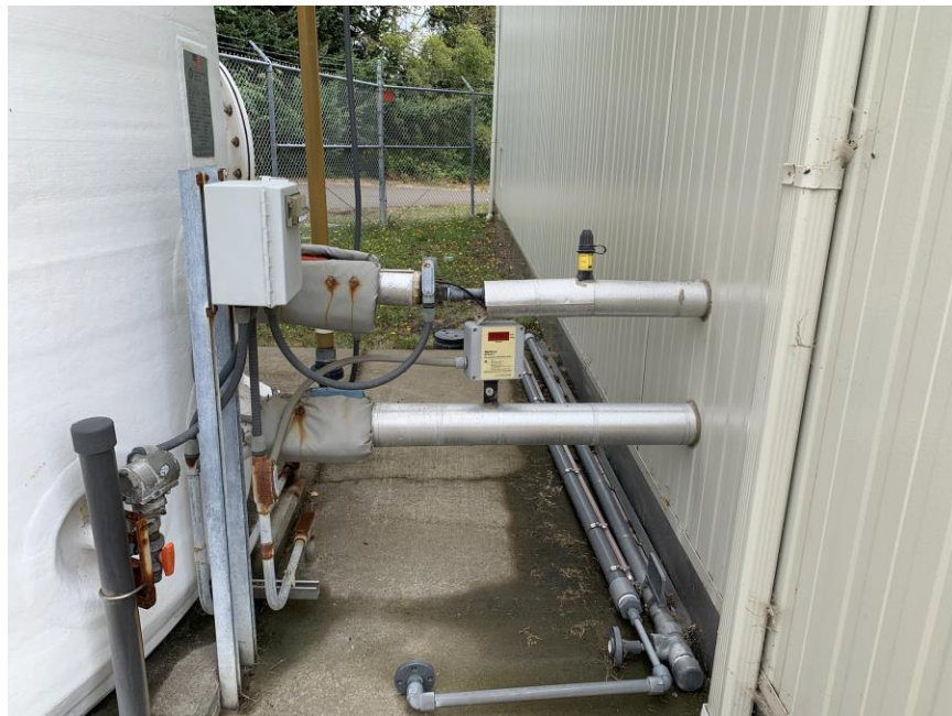
Figure 3.80 – Piping Connecting Salt Brine Tank to Sodium Hypochlorite Generation Building without Adequate Flexibility
