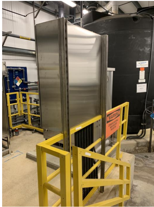
Figure 3.89 – Control Panel not Adequately Braced
