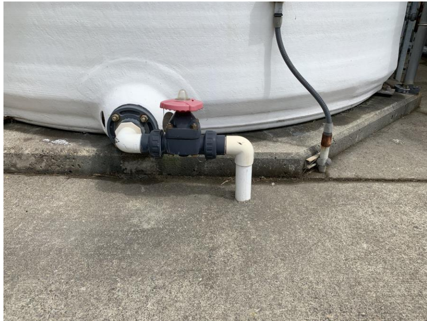
Figure 3.81 – Lack of Flexibility in Salt Brine Tank Drain Pipe
