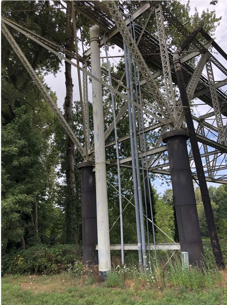
Figure 2. 24-inch Water Transmission Main
