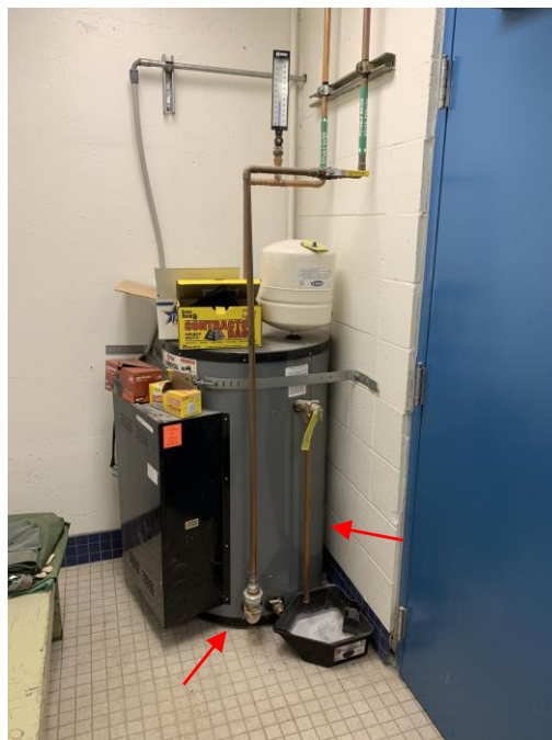
Figure 3.45 – Water Heater Tank not Adequately Restrained
