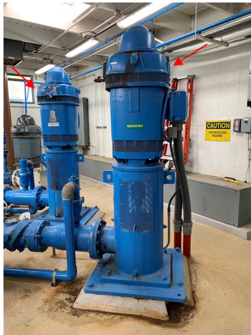
Figure 3.68 – Pump Motors not Braced to Structure Above their Center of Gravity
