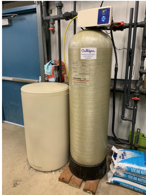
Figure 3.87 – Water Softener Components not Restrained
