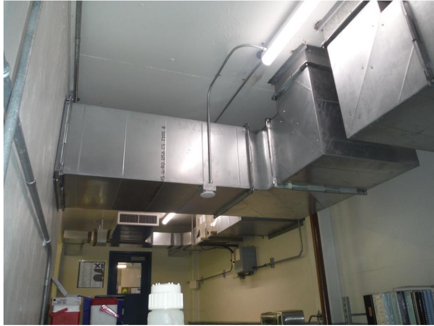
Figure 3.24 – Mechanical Ducts not Braced to Structure
