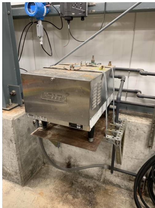
Figure 3.88 – Instant Hot Water Heater not Adequately Restrained
