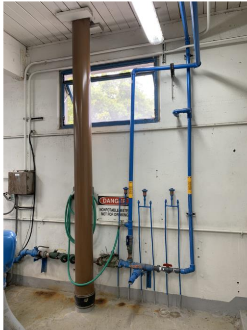
Figure 3.67 – Air Relief Piping Penetrating Laterally Unrestrained
