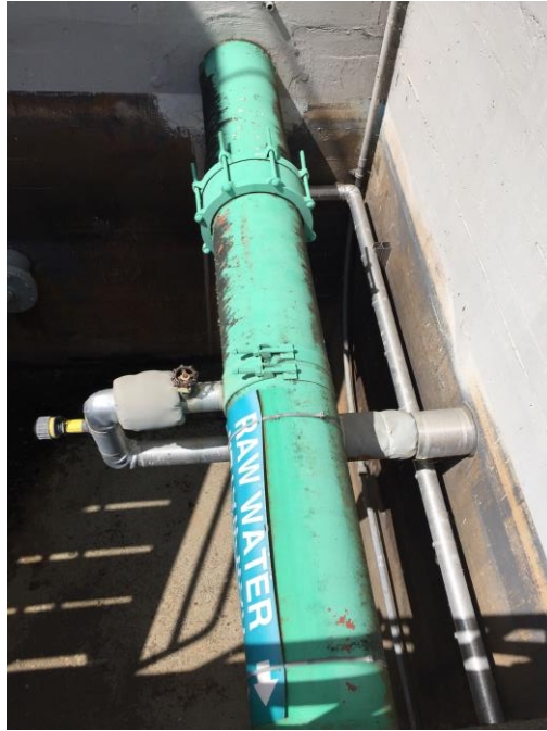
Figure 3.53 – Raw Water Pipes Penetrating Concrete Wall without Adequate Flexibility Through Wall
