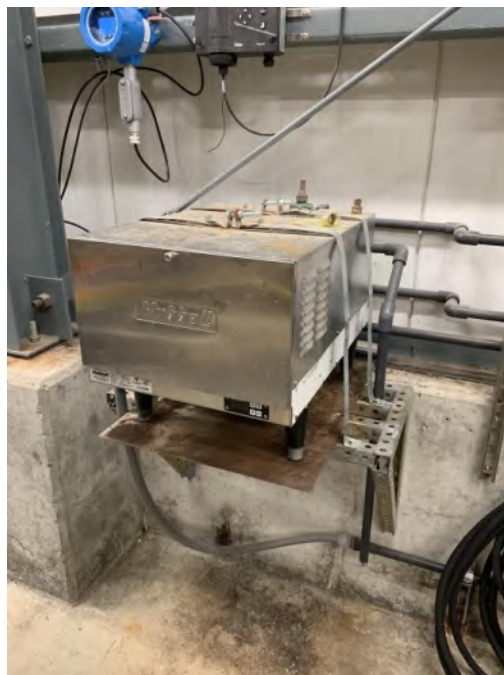
Figure 3.88 – Instant Hot Water Heater not Adequately Restrained
