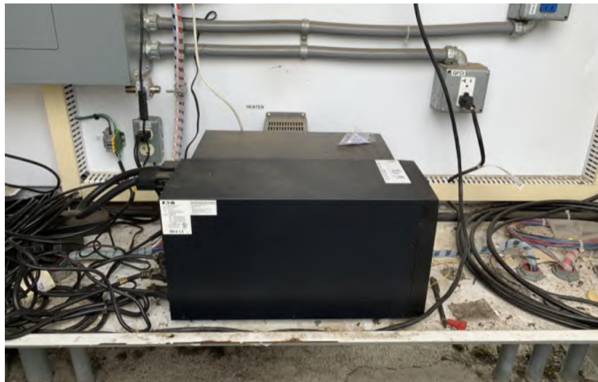
Figure 3.3 – Unrestrained Backup Batteries
