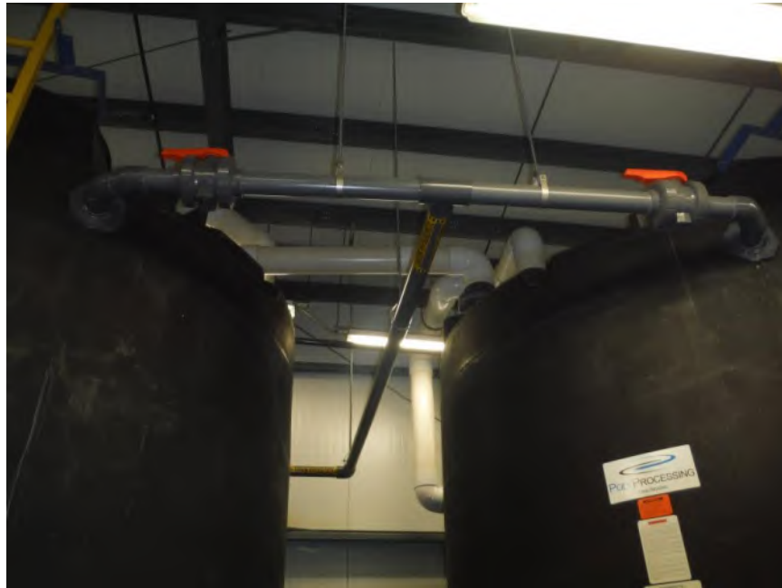
Figure 3.83 – Lack of Flexibility of Piping Connecting Sodium Hypochlorite Tanks
