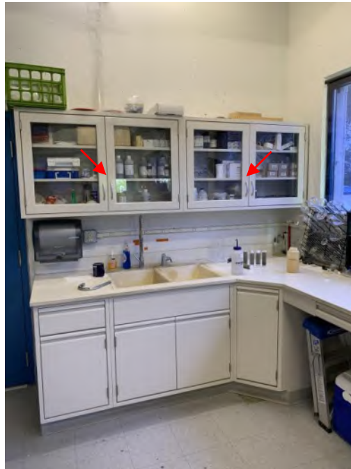
Figure 3.44 – Chemical Cabinet Doors without Proper Latches
