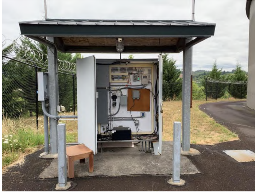
Figure 3.2 – Electrical Panelboard and SCADA Equipment Enclosure and Canopy
