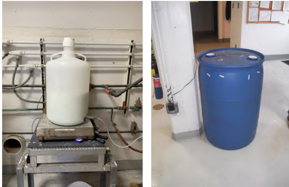
Figure 3.20 – Unrestrained Chemical Storage Containers
