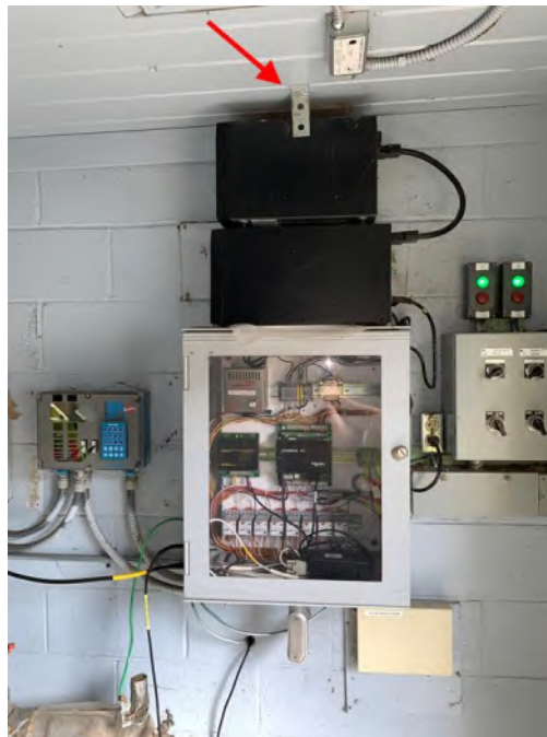
Figure 3.9 – Backup Batteries not Adequately Restrained
