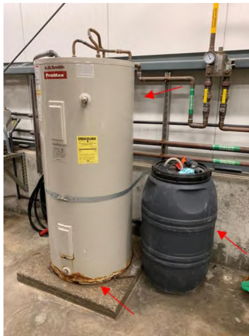
Figure 3.86 – Water Heater not Adequately Restrained and Unrestrained Barrel
