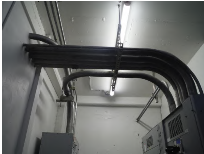
Figure 3.26 – Electrical Conduits not Seismically Braced and without Flexible Connections to Cabinets
