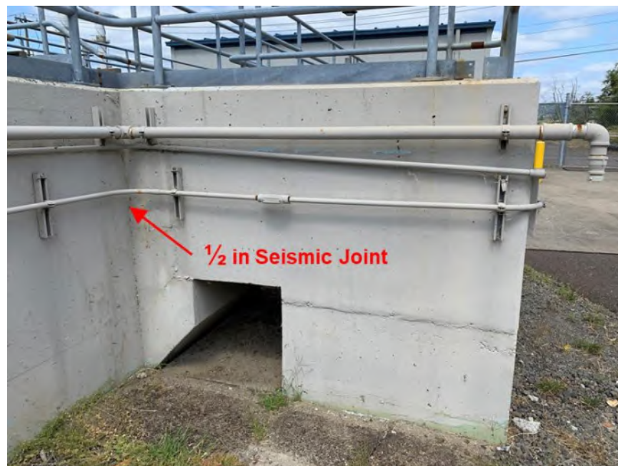
Figure 3.50 – Sedimentation Basins Effluent Structure (Outlet Basin Structure)
