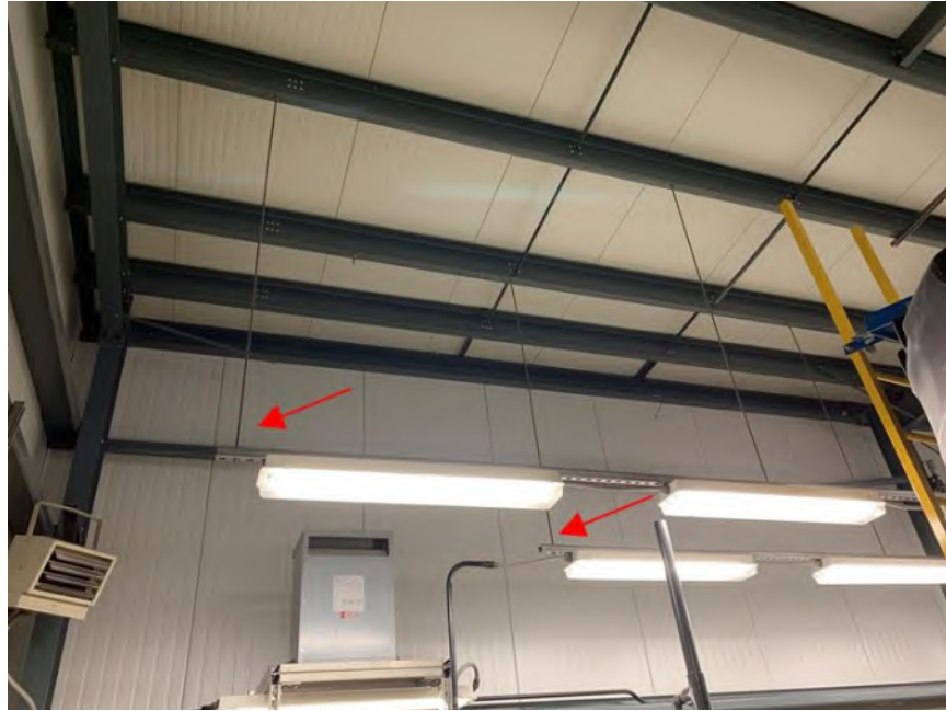
Figure 3.91 – Unrestrained Light Fixtures
