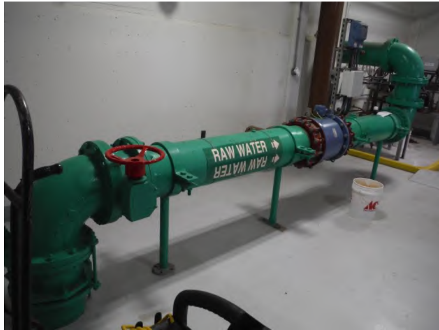
Figure 3.18 – Raw Water Piping System without Adequate Bracing
