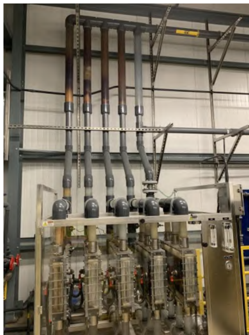
Figure 3.84 – Lack of Flexibility in Piping between Sodium Hypochlorite Generator and Attachment to Building
