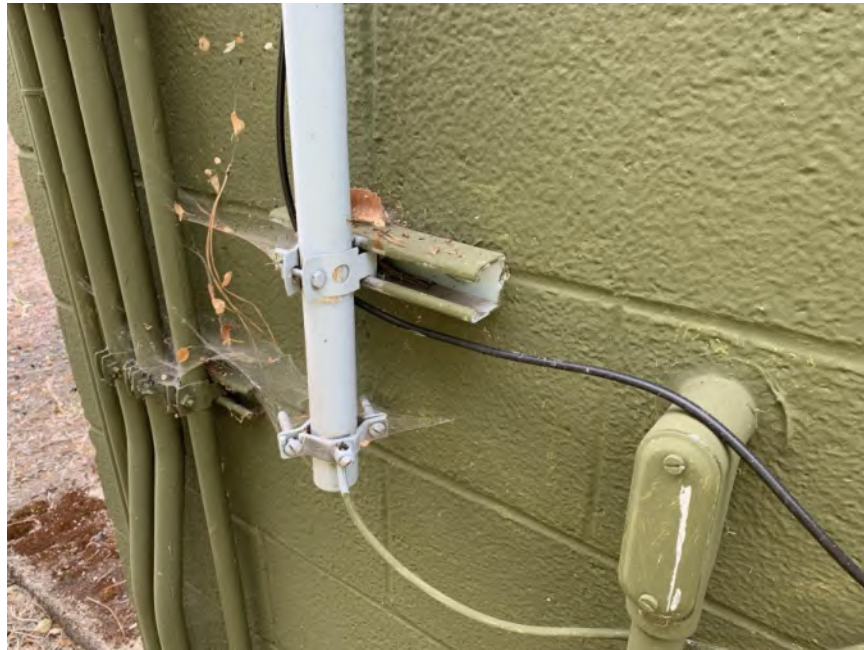
Figure 3.10– SCADA Antenna Supported with Friction Clips
