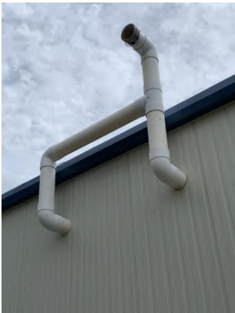
(a) Unbraced Piping Outside the Building
