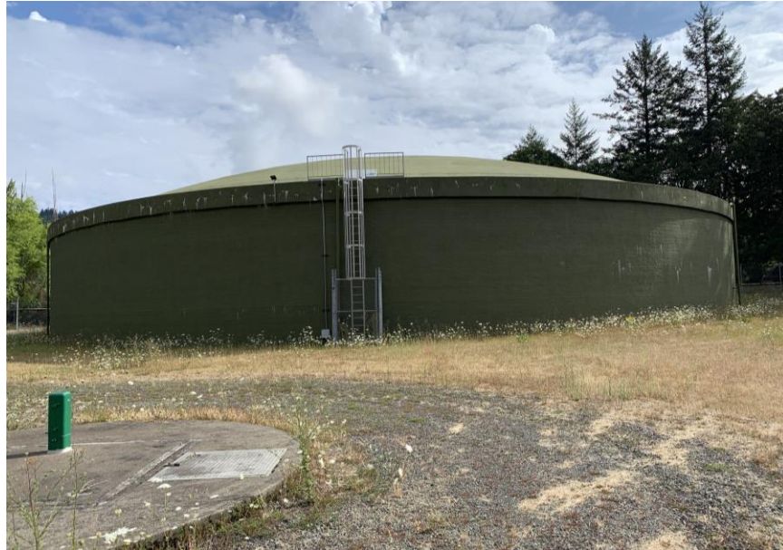
Figure 3.11 – North Valley Reservoir No.2
