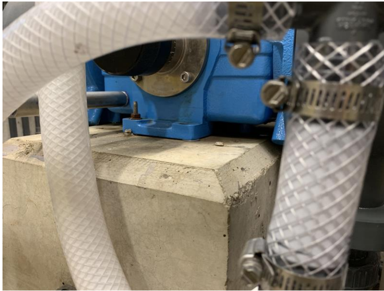
Figure 3.85 – Deficient Anchorage Between Chemical Feed Pumps and Concrete Support
