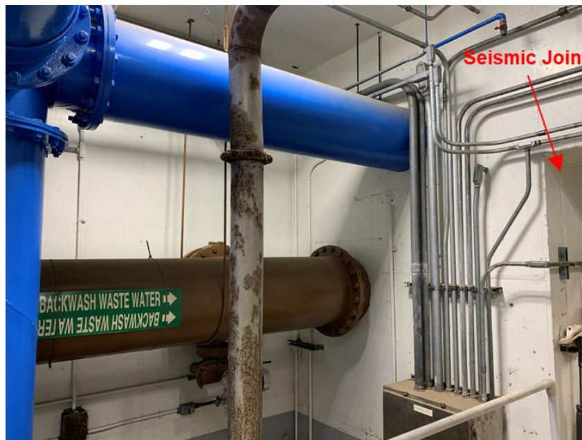
Figure 3.62 – Finished Water Sample Pipe and Filter Backwash Pipe Cross Seismic Joint without Adequate Flexibility
