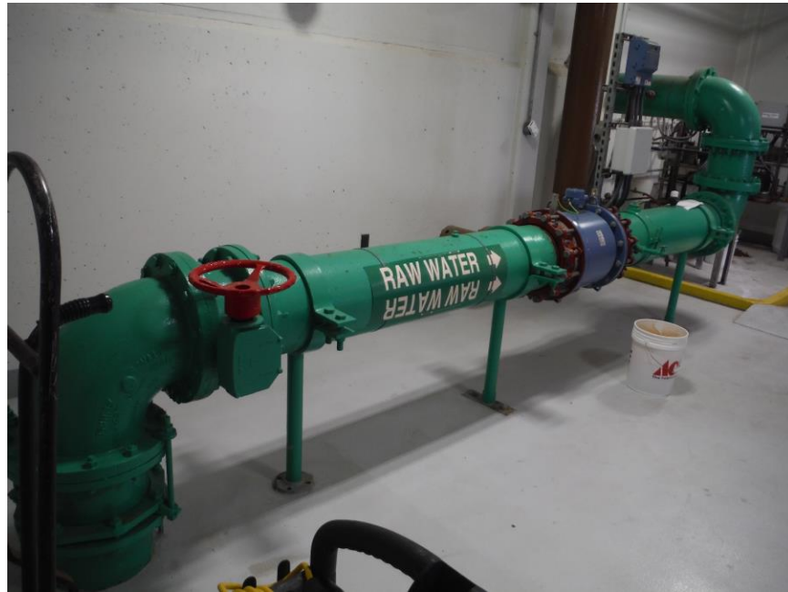
Figure 3.18 – Raw Water Piping System without Adequate Bracing
