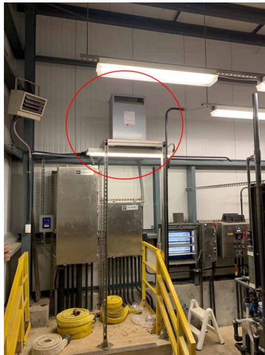
Figure 3.90 – Transformer not Adequately Braced
