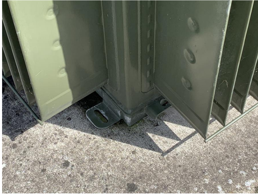
Figure 3.96 – Electrical Transformer not Anchored to Concrete Pad
