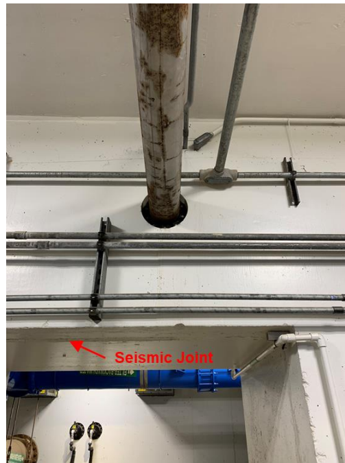
Figure 3.63 – Air Scour Pipe Crosses Seismic Joint without Adequate Flexibility
