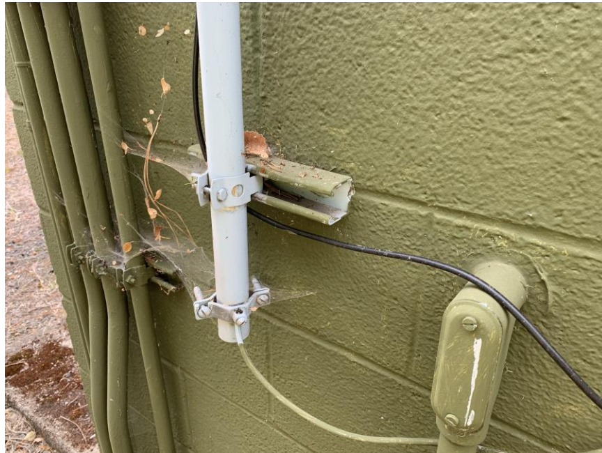
Figure 3.10– SCADA Antenna Supported with Friction Clips
