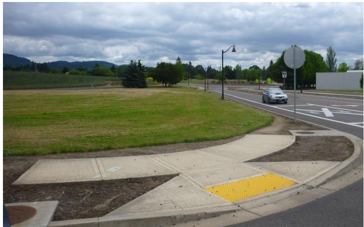
ADA Compliant Curb Ramp with No Connections
