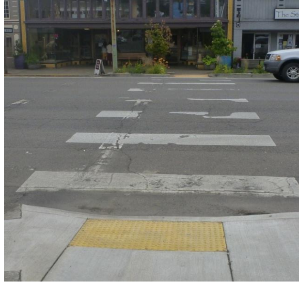
Faded Crosswalk in Downtown Newberg
