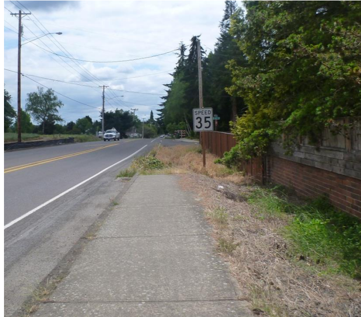
Gaps in Sidewalks on Arterial Roadway
