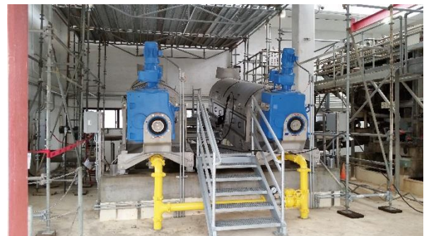
Figure 3: Screw Presses Installed
