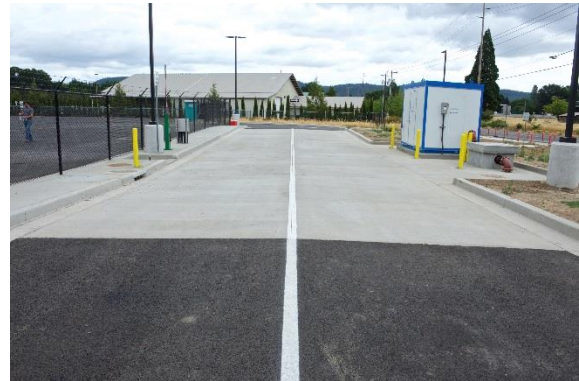
Figure 4: Septage Receiving & RV Dump Station expanded capacity and increased functionality at the wastewater treatment plant.
